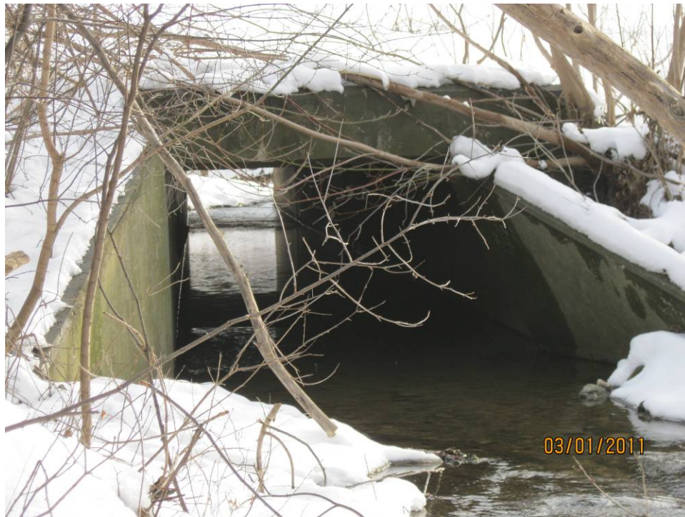
Photo 13: The downstream end of the culvert under Indiana Avenue. Note the recently collapsed wing wall.
