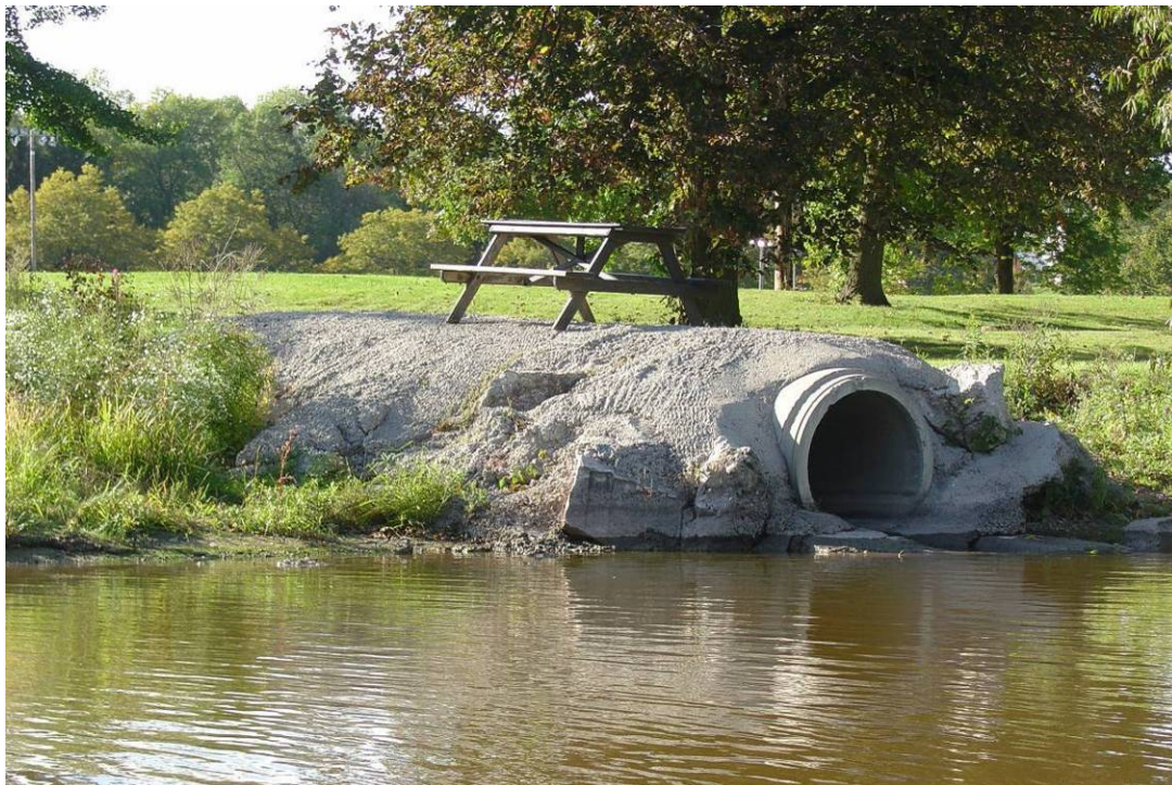
Photo 8: Another stormwater outfall along the shoreline that has been cemented in place due to erosion.
