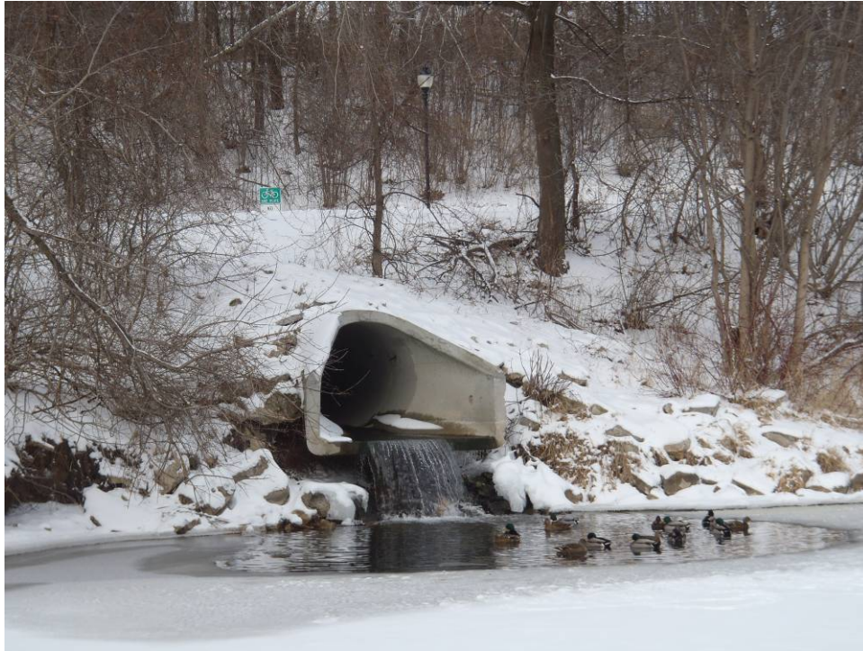
Photo 7: Largest stormwater outfall at Kiwanis Park, which creates a large scour hole.
