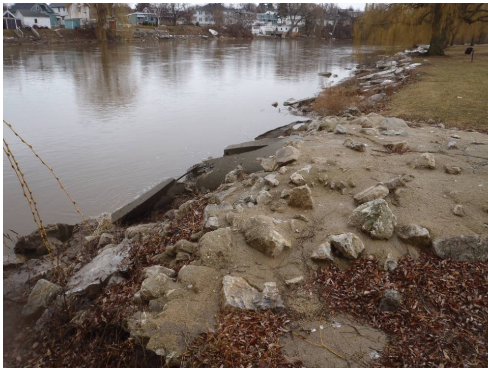
Photo 6: A damaged stormwater outfall, concrete and other rip-rap along shoreline.
