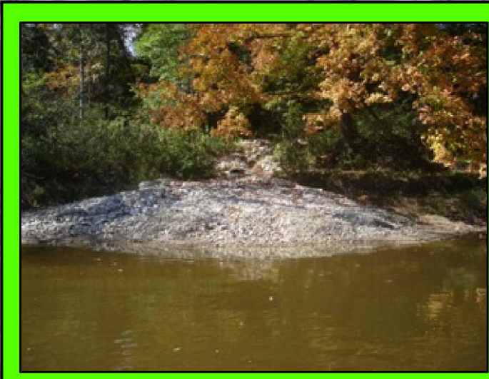
Bank Stabilization - Culvert Erosion
