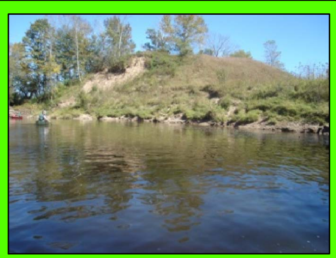
Bank Stabilization - Bank Sloughing at Kohler
