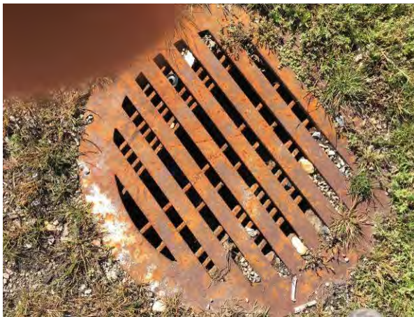
Photo #9 Storm sewer inlet full of water on eastern portion of the Parcel
