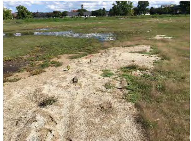
Photo #14 Small pile of crushed limestone and ponded water – looking east
