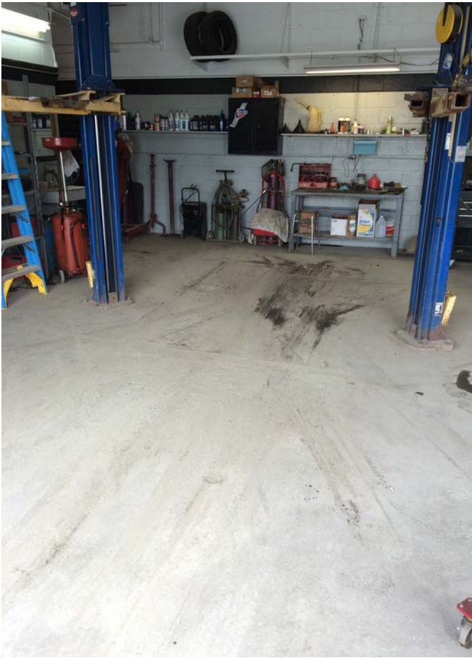
#5 - View of hydraulic lift system #2, looking east
