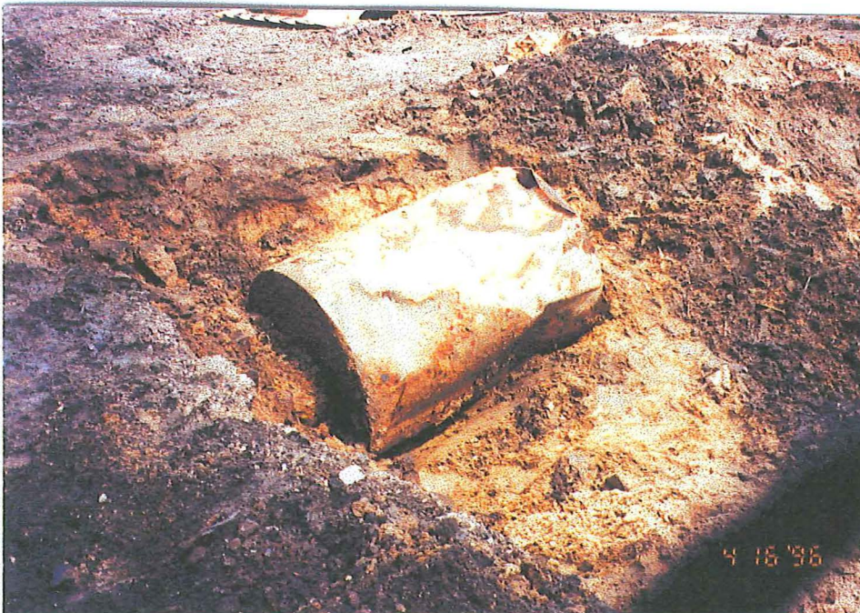
View of the approximately 500 gallon underground storage tank.
