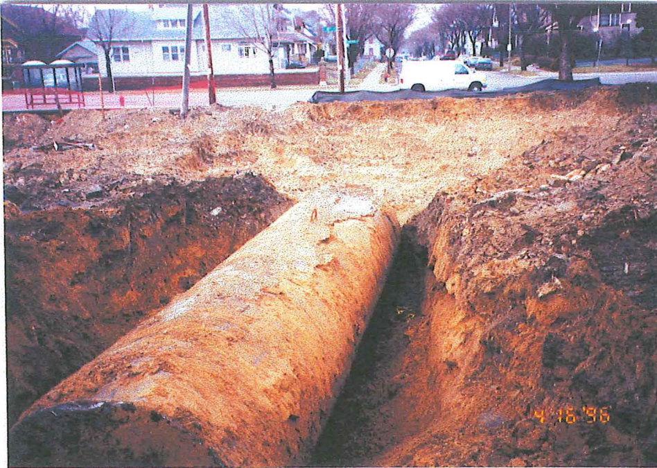
View toward the south of two approximately 4,000 gallon underground storage tank. The side of the other tank is visible to the west (right) of the completely exposed tank.
