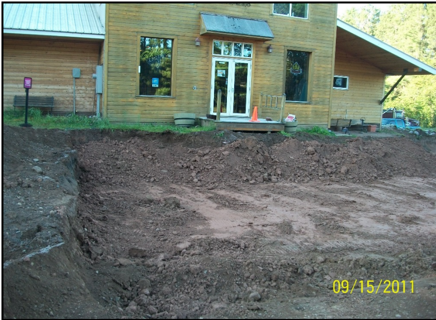
View of structural impediment from north
