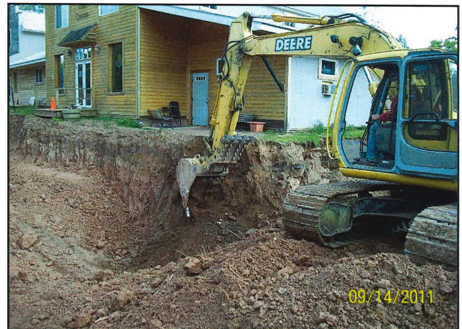
View of structural impediment from northwest
