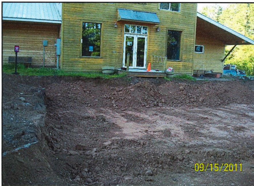
View of structural impediment from north
