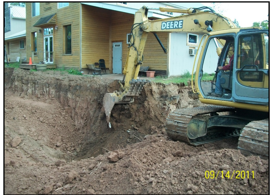
View of structural impediment from northwest
