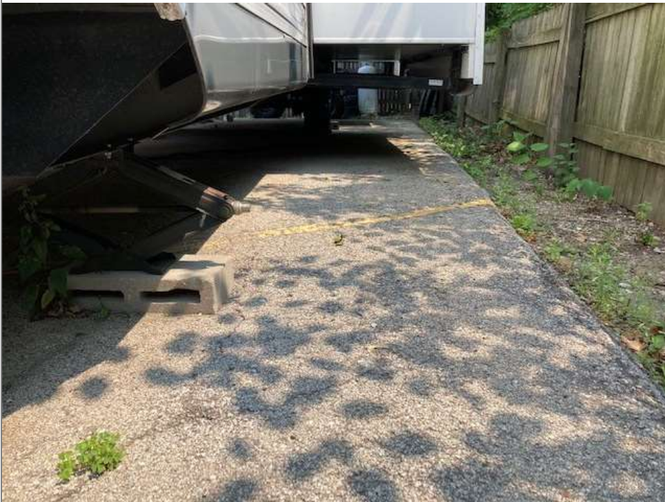
Title: South end of pavement along the south property line, facing east.
