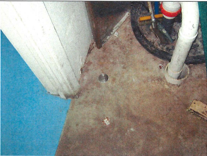
Photo 33: Flush mount cap at SSV-9.
