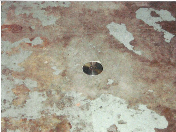
Photo 5: Flush mount cap at SSV-3.
