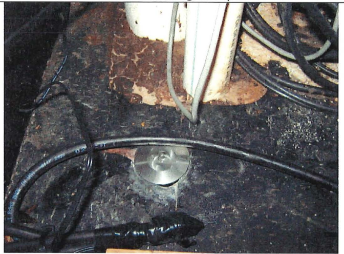
Photo 28: Flush mount cap at SSV-6.
