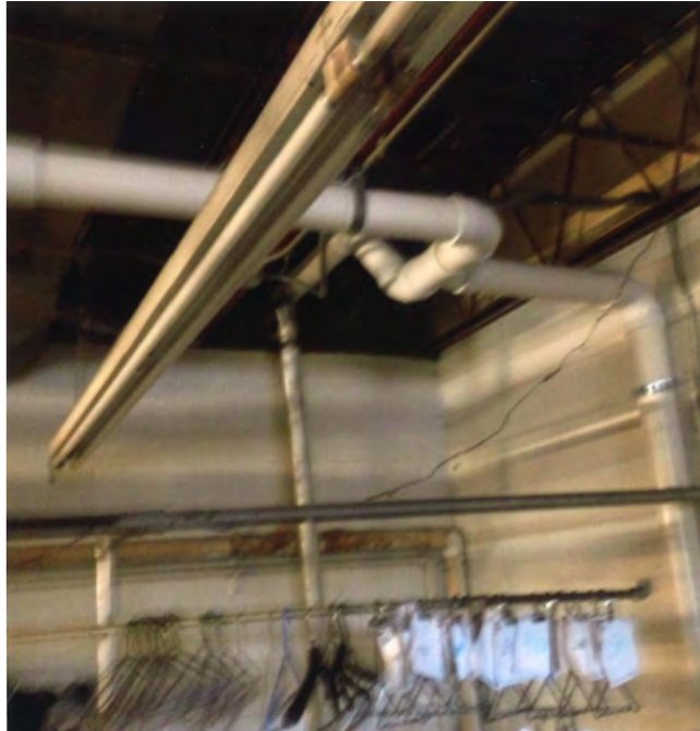
Photo 1: Piping where two pickup points join in Donaldson's One Hour Cleaners.
