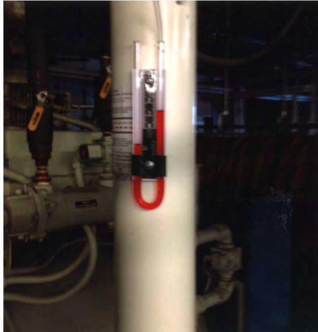
Photo 3: Manometer on first pickup point in Donaldson's One Hour Cleaners.
