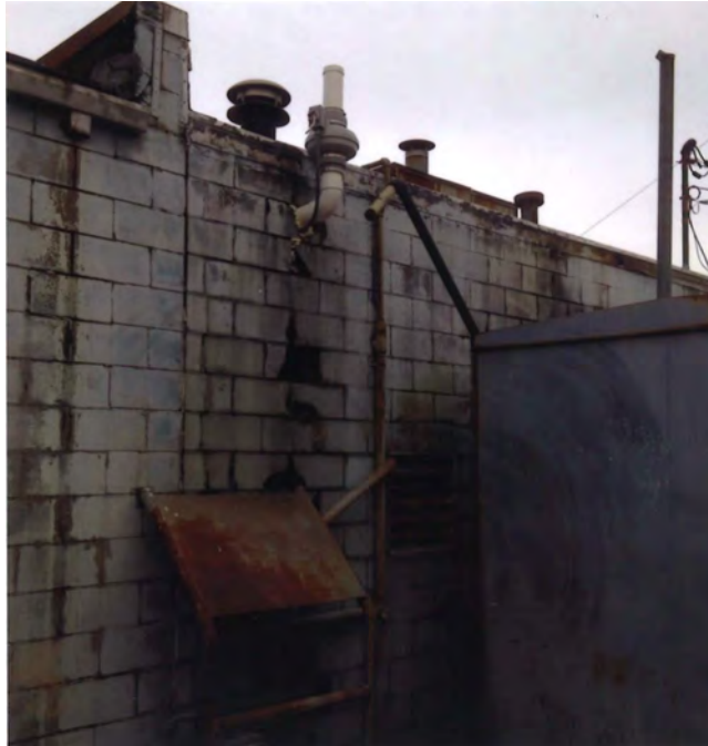
Photo 5: Fan and discharge behind Donaldson's One Hour Cleaners.
