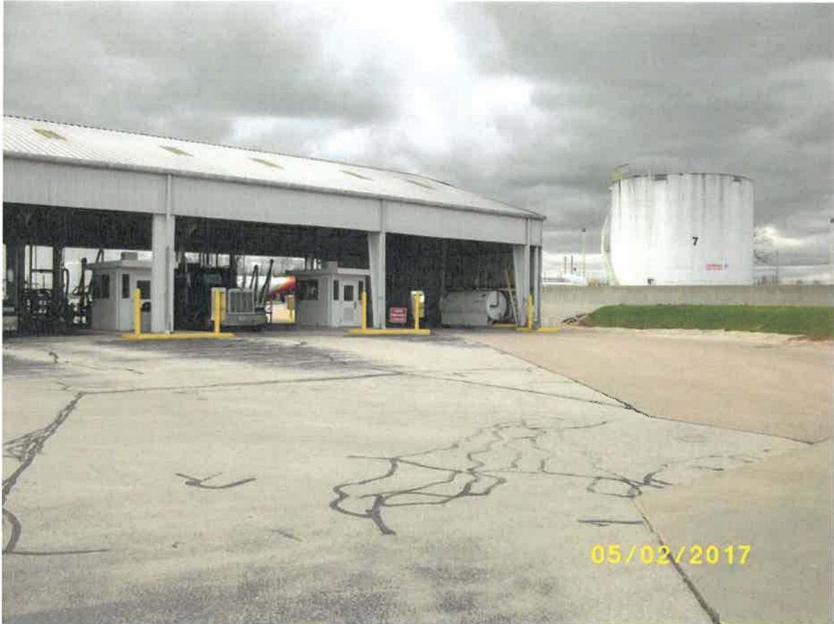
Structural Impediment (View Northwest)
