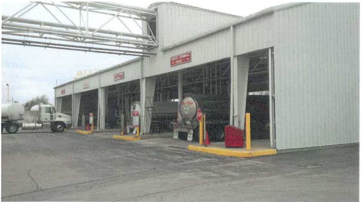
Photograph 1 – Structural Impediment (View Northeast)
