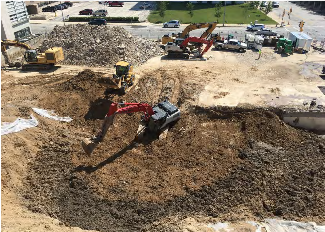
Photo 5: Blending stockpiled slope and access ramp soils into the top five feet of the treatment area. Photograph looking east.
