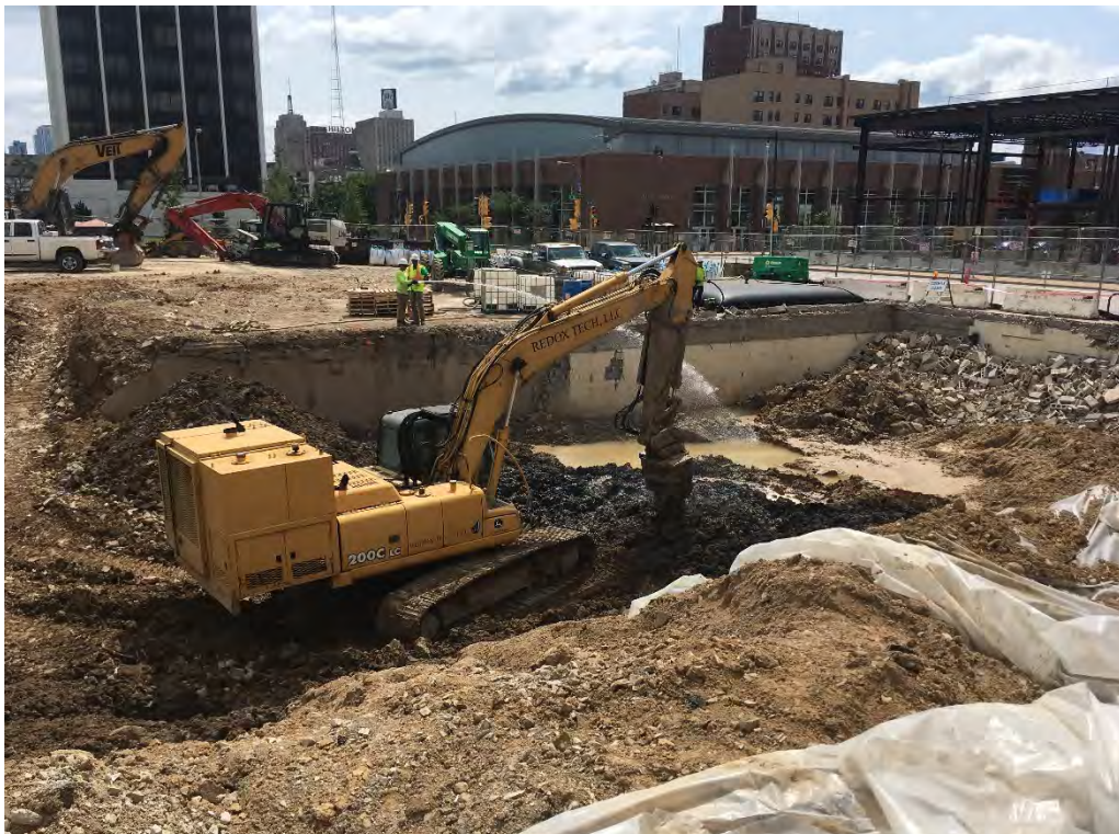
Photo 2: Soil blending and chemical amendment application within treatment cell 4. Photograph looking east-southeast.
