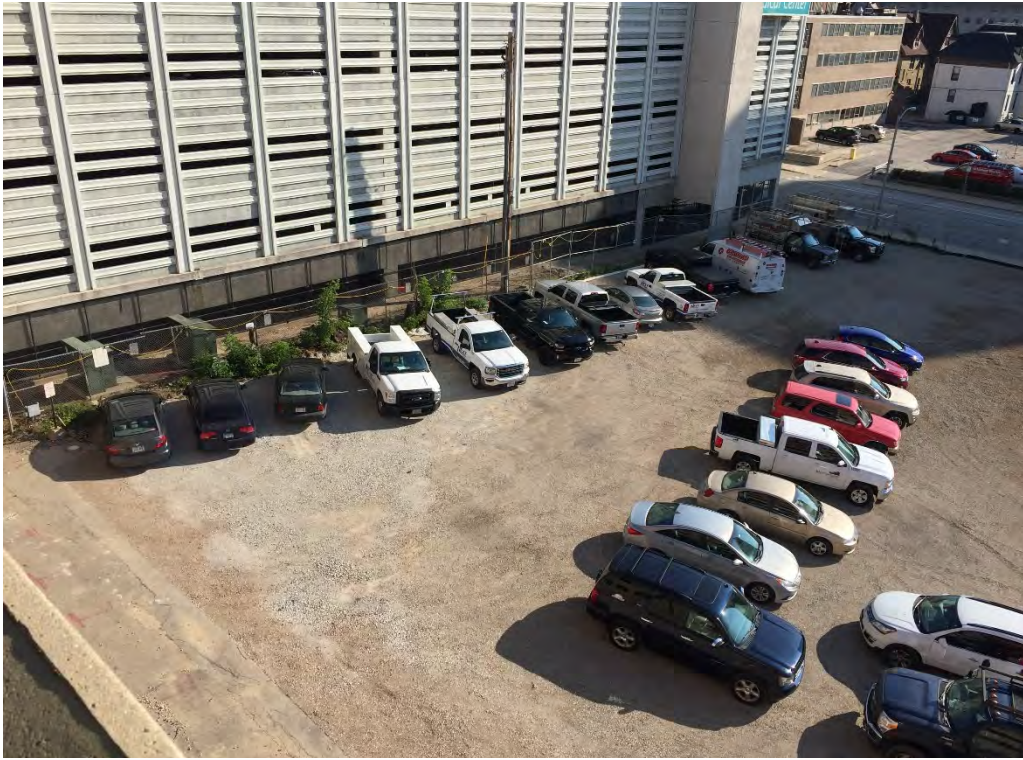
Photo 7: Completed backfilling and compaction activities of soil treatment area. Photograph looking northeast.
