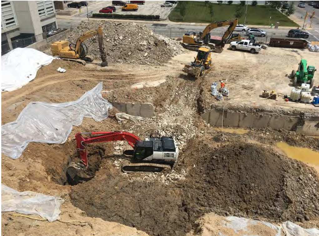
Photo 1: Excavating treatment cell 2 and preparing to blend chemical amendments. Covered stockpiled slope and access ramp soils in background-left. Photograph looking east.
