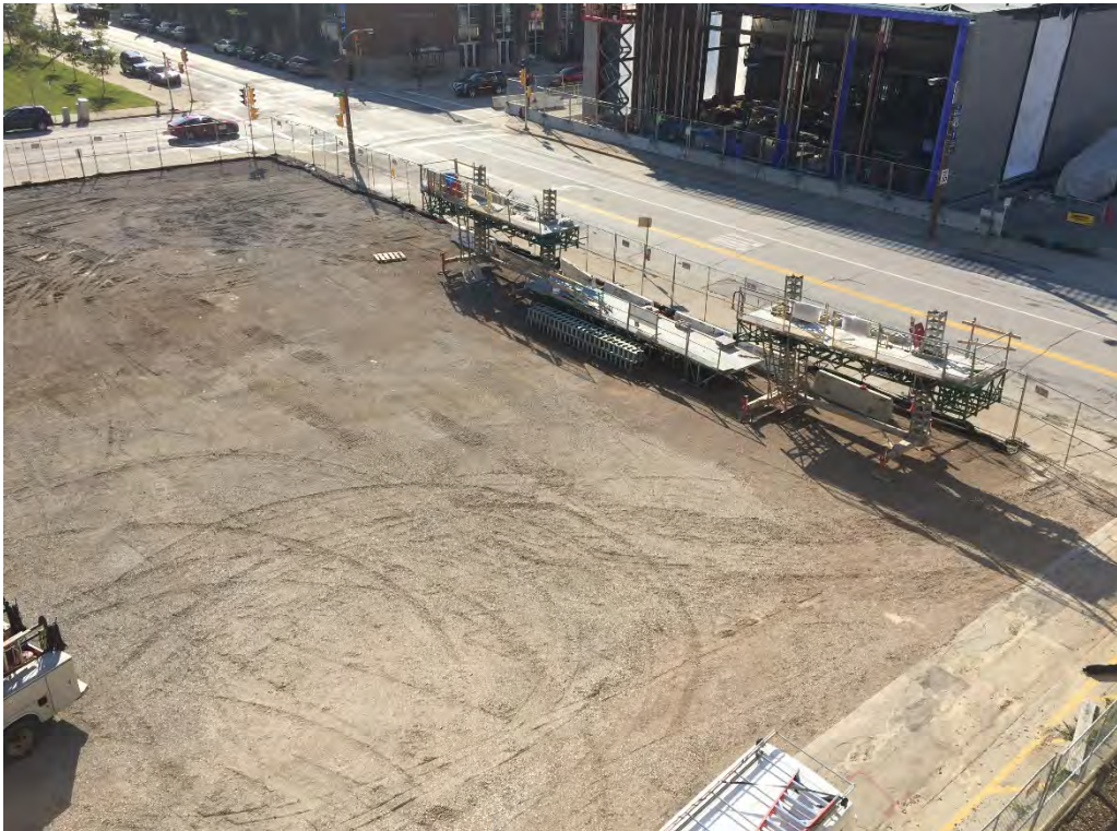
Photo 8: Completed backfilling and compaction activities of soil treatment area. Photograph looking southeast.
