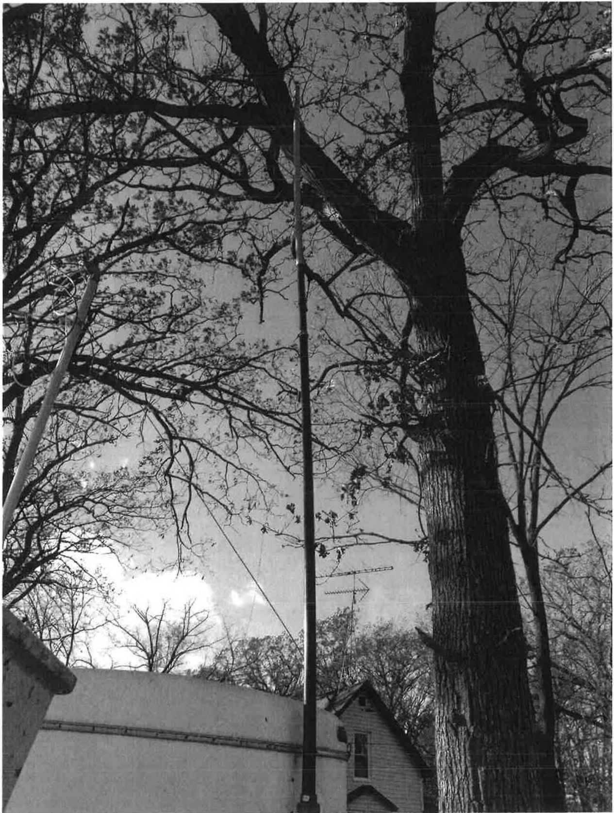
Photo 3 - Photo showing the November stack height extension (white segment at top of pipe). Pipe is braced against tree to stabilize it.
