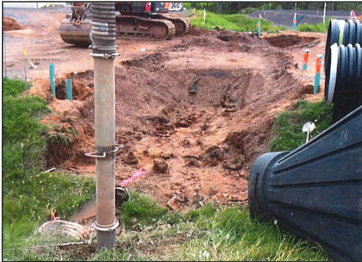
Photo 5: Culvert removal trench. The historical culvert is visible near the bottom of the vertical hydrovacuum truck metal hose in the bottom left corner of the photo. Photo taken facing southeast on November 15, 2014.
