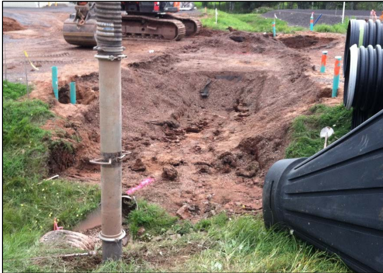
Photo 5: Culvert removal trench. The historical culvert is visible near the bottom of the vertical hydrovacuum truck metal hose in the bottom left corner of the photo. Photo taken facing southeast on November 15, 2014.
