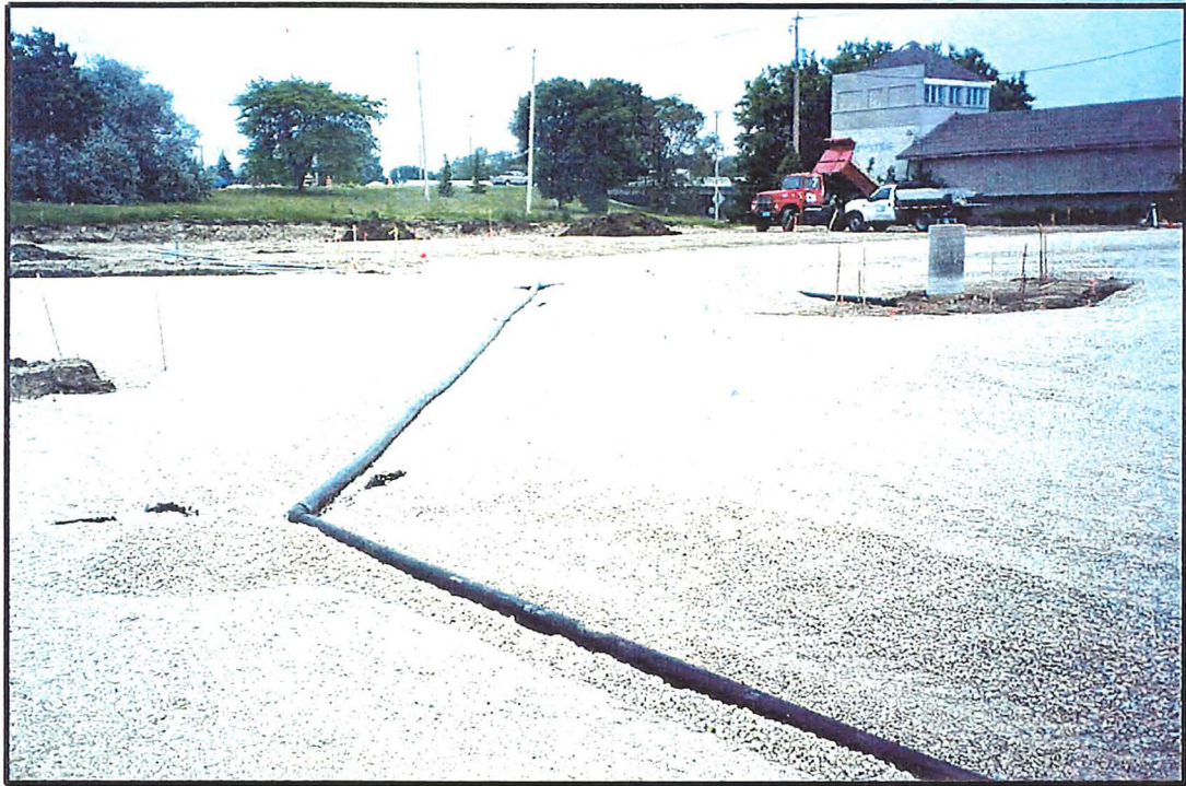
Installed parking lot passive gas venting system.
