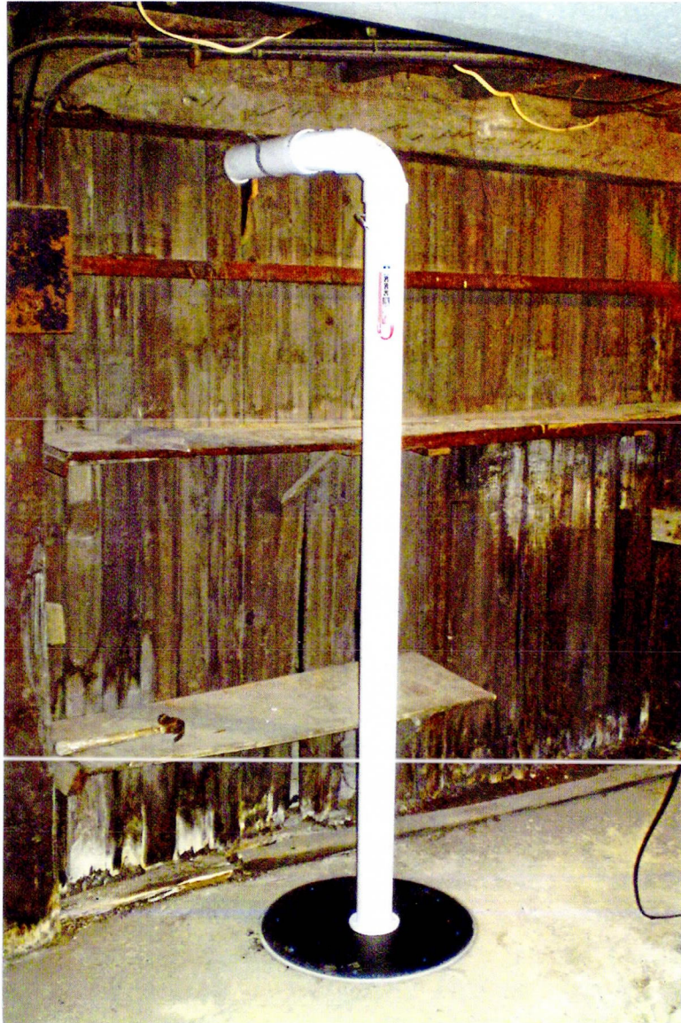
Photo 1: Main pick-up point (P2), located near the middle of the building. Vapor mitigation system installed February 6, 2014, by Acura Services, LLC.
