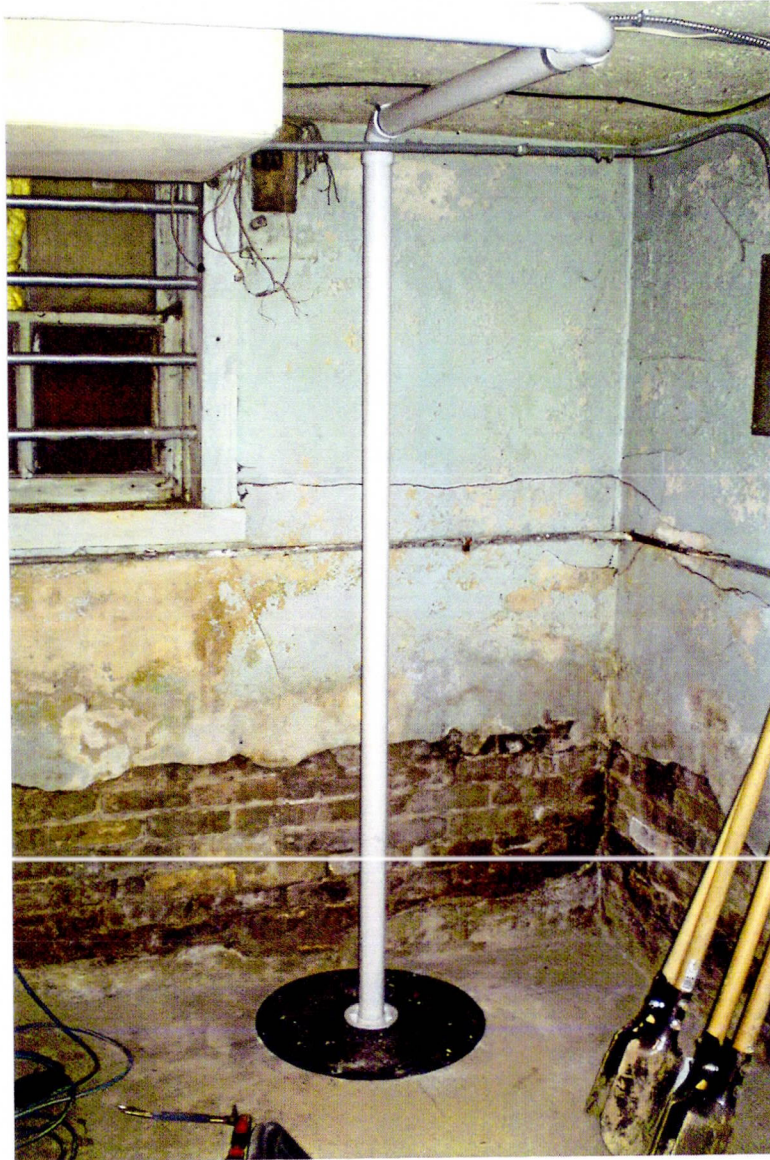
Photo 2: Pick-up point (P3), located nearest the source, southwest corner of the building. Vapor mitigation system installed February 6, 2014, by Acura Services, LLC.
