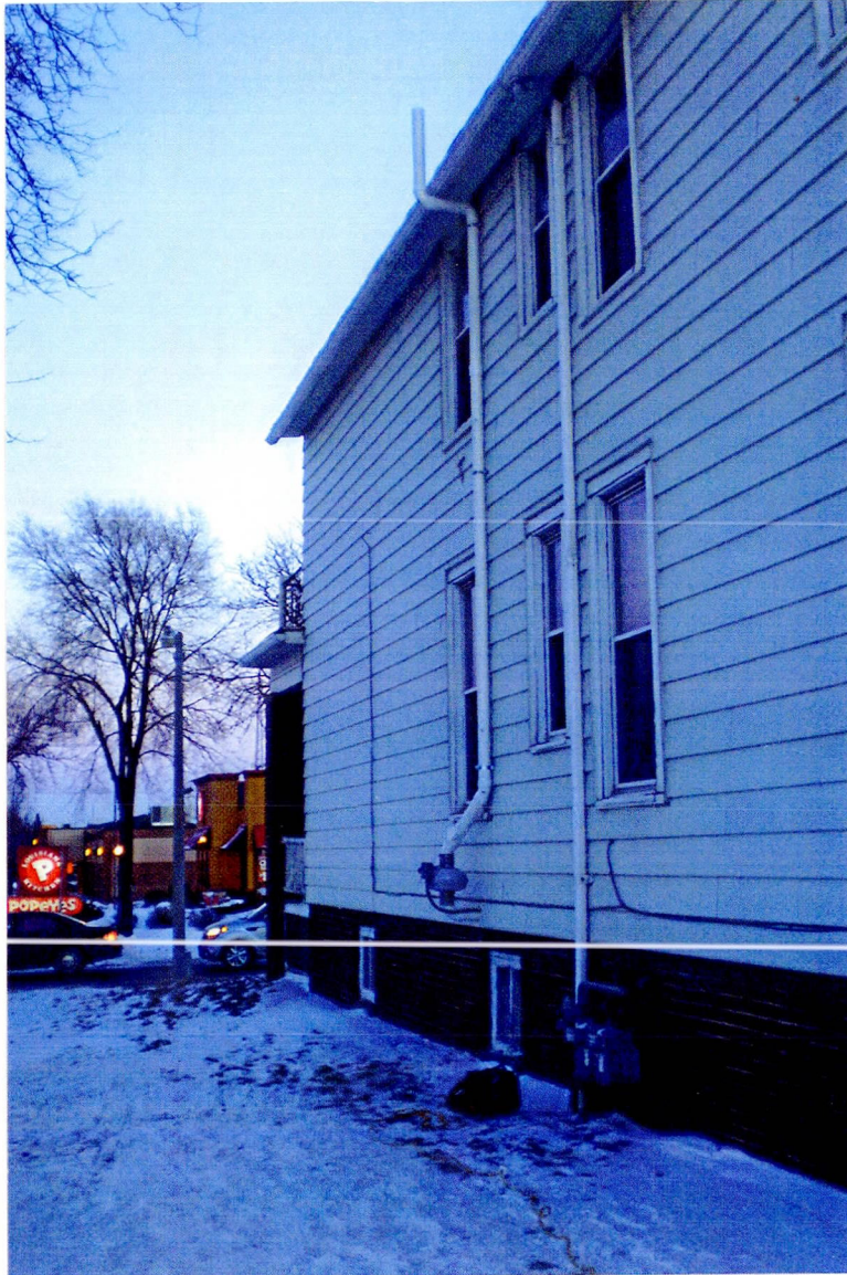
Photo 3: Vent pipe located on the north side of the building. Vapor mitigation system installed February 6, 2014, by Acura Services, LLC.
