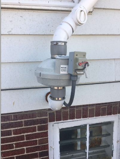
Title: Fan on north side of house - red switch in "on" position
