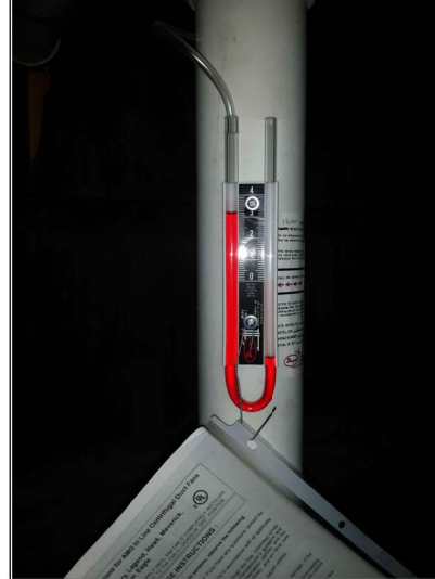
Title: Manometer located at P2 shown with deflection - fan operating
