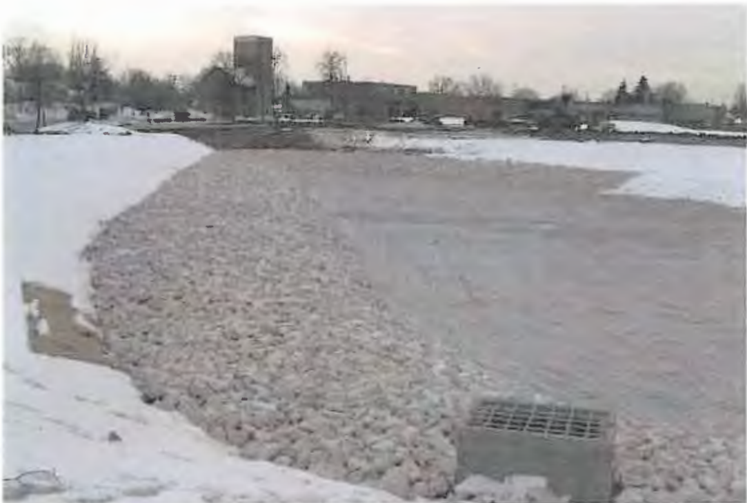
PHOTOGRAPH 38: Wet Detention Pond Installation: Stone and topsoil completion, photograph taken looking south.
