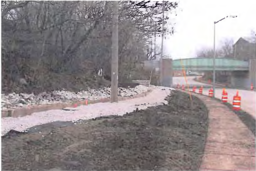
PHOTOGRAPH 31: Interceptor Trench Installation: Interceptor trench installation and berm construction along West Becher Place, photograph taken looking north.
