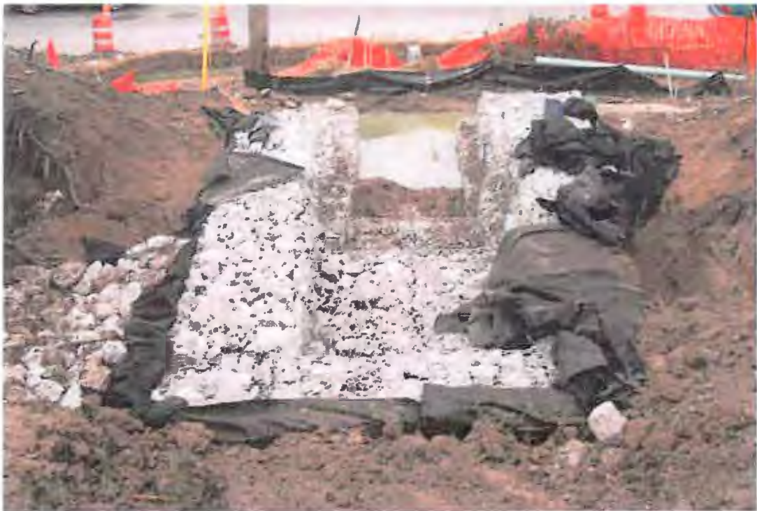
PHOTOGRAPH 10: Stormwater Controls: Gabion-lined channel construction, ditch check located along West Becher Place easement.
