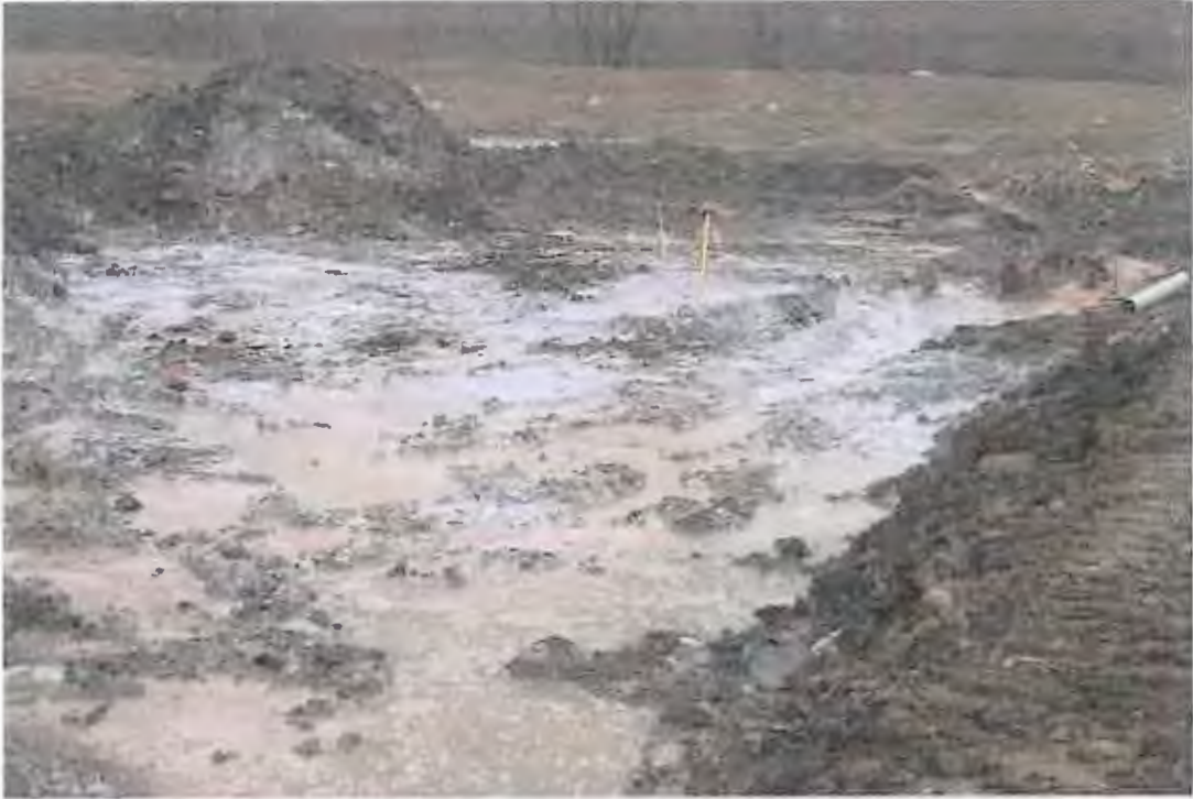
PHOTOGRAPH 33: Wet Detention Pond Installation: Pond excavation, bridge lift subgrade, photograph taken looking north.
