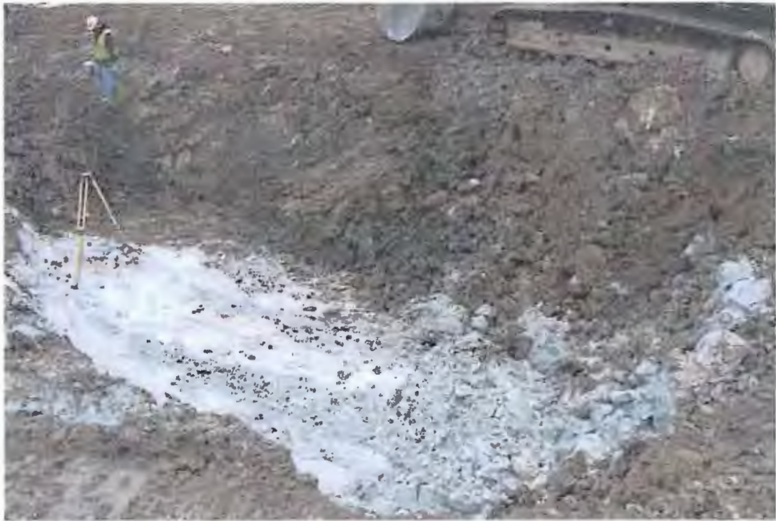
PHOTOGRAPH 27: Site Grading and Earthwork: Wet detention pond excavation, over excavation extent for bridge lift subbase.
