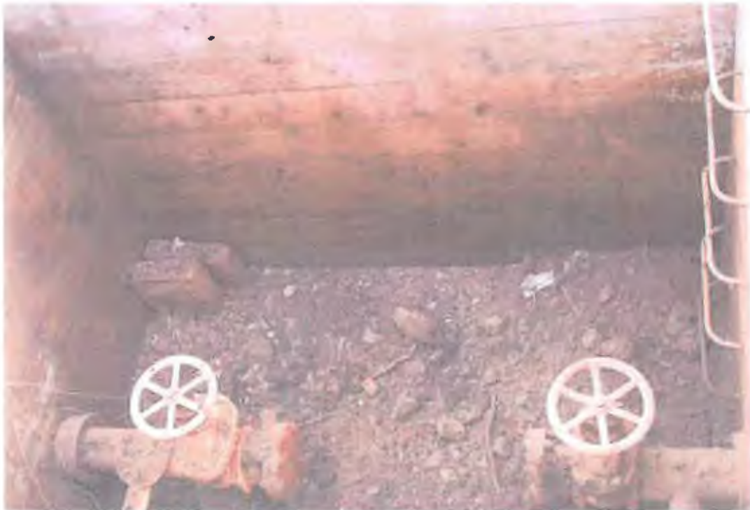
PHOTOGRAPH 16: Second Sprinkler Vault: Access piping abandoned as shown. Site piping, valve, and concrete structure removed per specifications.
