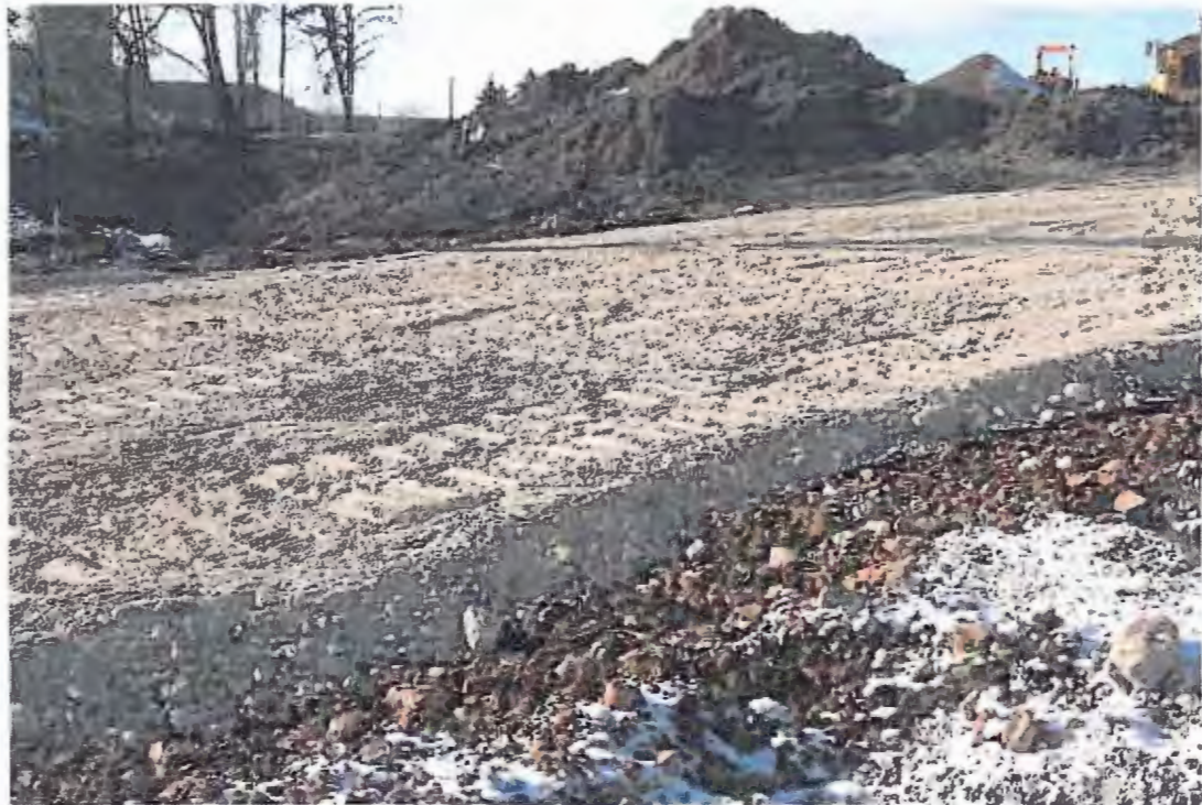
PHOTOGRAPH 40: Site Restoration: Stabilized gravel entrance, West Becher Place access road, photograph taken looking southeast.
