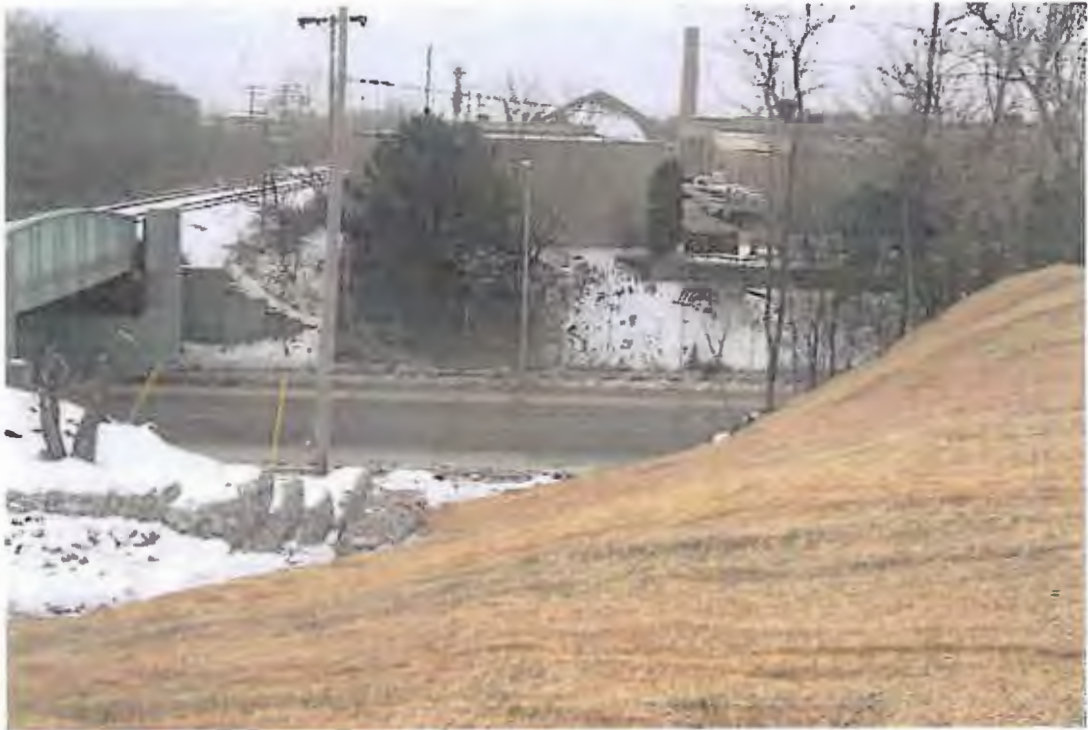
PHOTOGRAPH 29: Gabion-Lined Channel: Gabion-lined channel complete with slope restoration, photo taken looking east.
