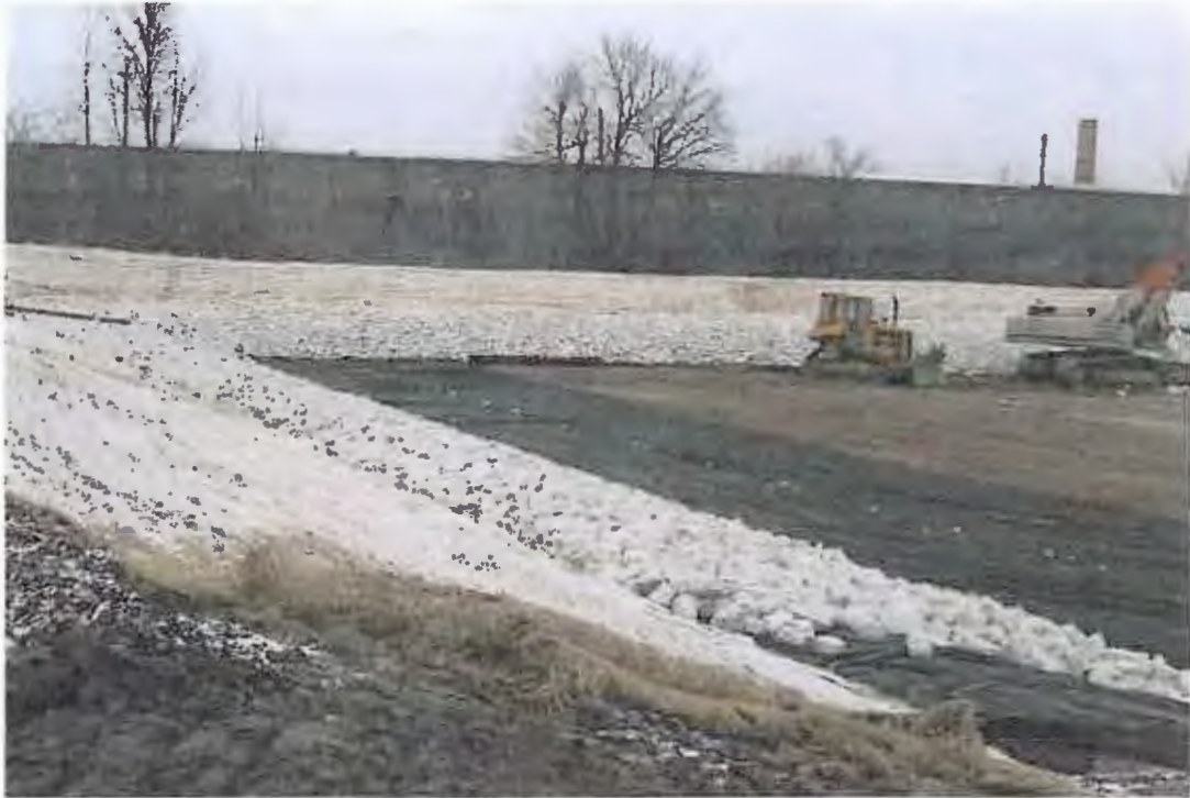
PHOTOGRAPH 37: Wet Detention Pond Installation: Topsoil and stone placement, photograph taken looking north.
