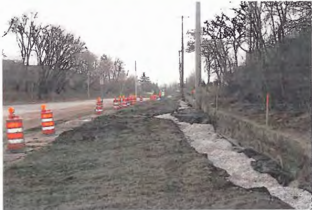
PHOTOGRAPH 30: Interceptor Trench Installation: Interceptor trench installation along West Becher Place, photograph taken looking south.
