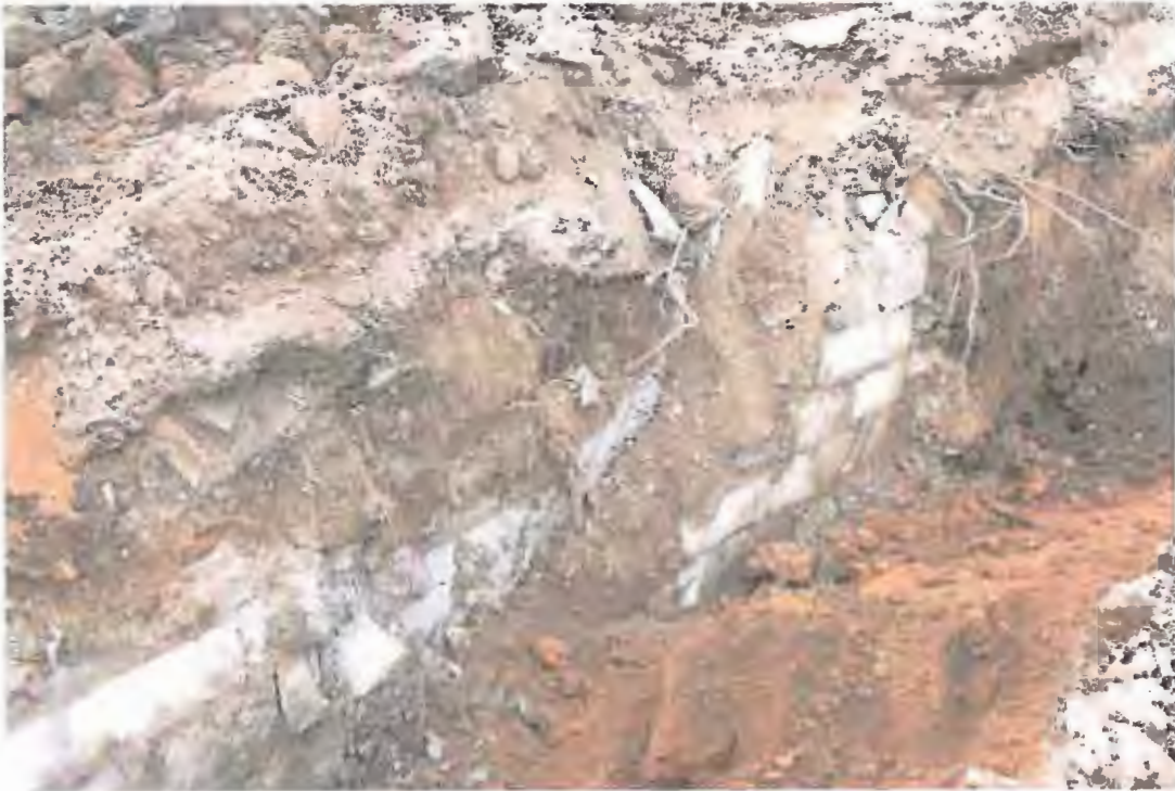
PHOTOGRAPH 17: Sprinkler Vault: Retaining wall exposed during discharge pipe abandonment. Wall crushed in place to five feet below ground surface per specifications.
