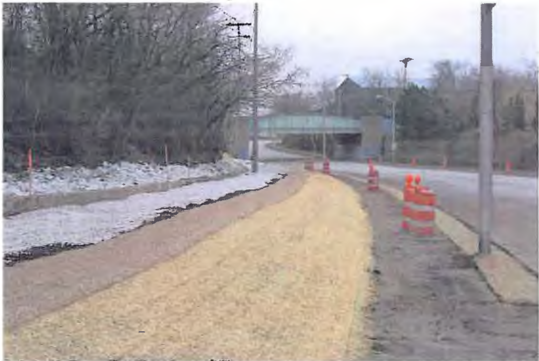
PHOTOGRAPH 32: Interceptor Trench Installation: Interceptor trench berm construction along West Becher Place, photograph taken looking north.
