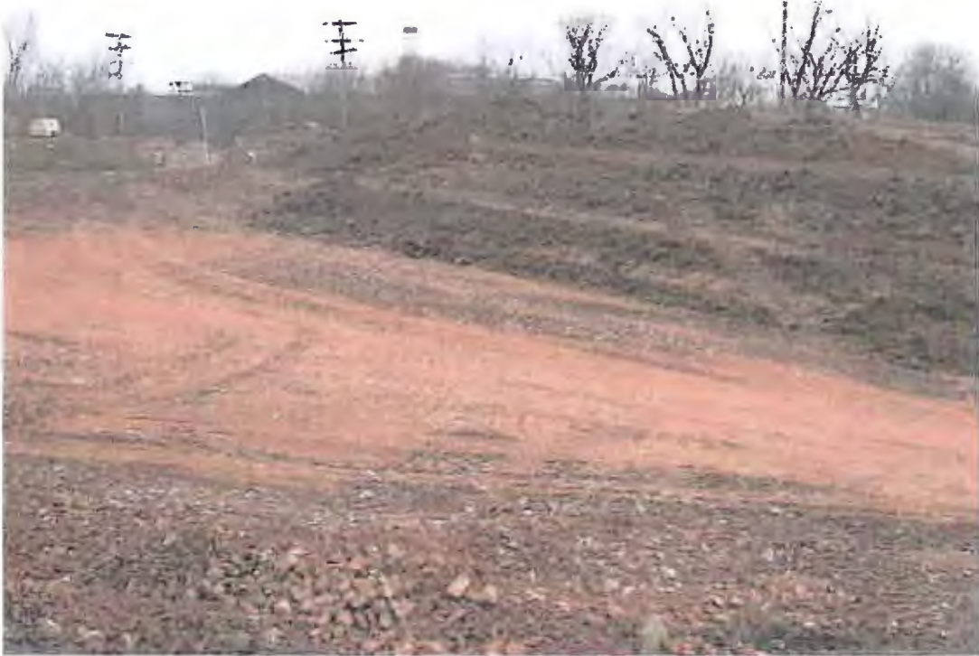
PHOTOGRAPH 35: Wet Detention Pond Installation: Bridge lift construction, bridge lift and clay liner installation, photograph taken looking northeast.
