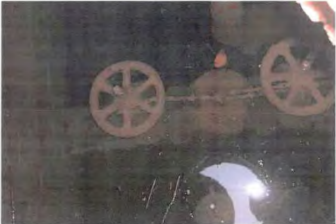
PHOTOGRAPH 14: Sprinkler Vault: Water pumped and disposed of offsite, piping and concrete structure removed per specifications.
