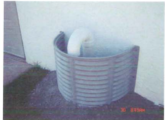
Photo 4 Exterior Vapor Venting
