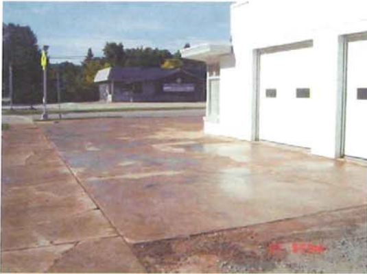
Photo 1 Western Concrete Cover
