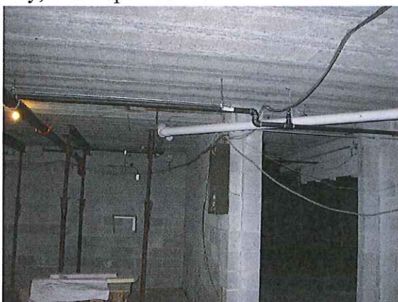
White PVC vent pipe along ceiling.
