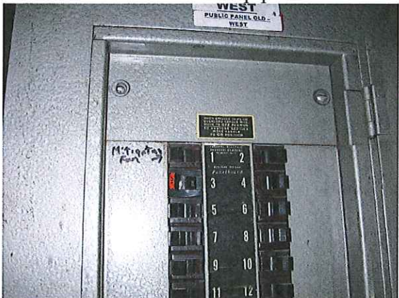
Dedicated breaker switch (#1) on.
