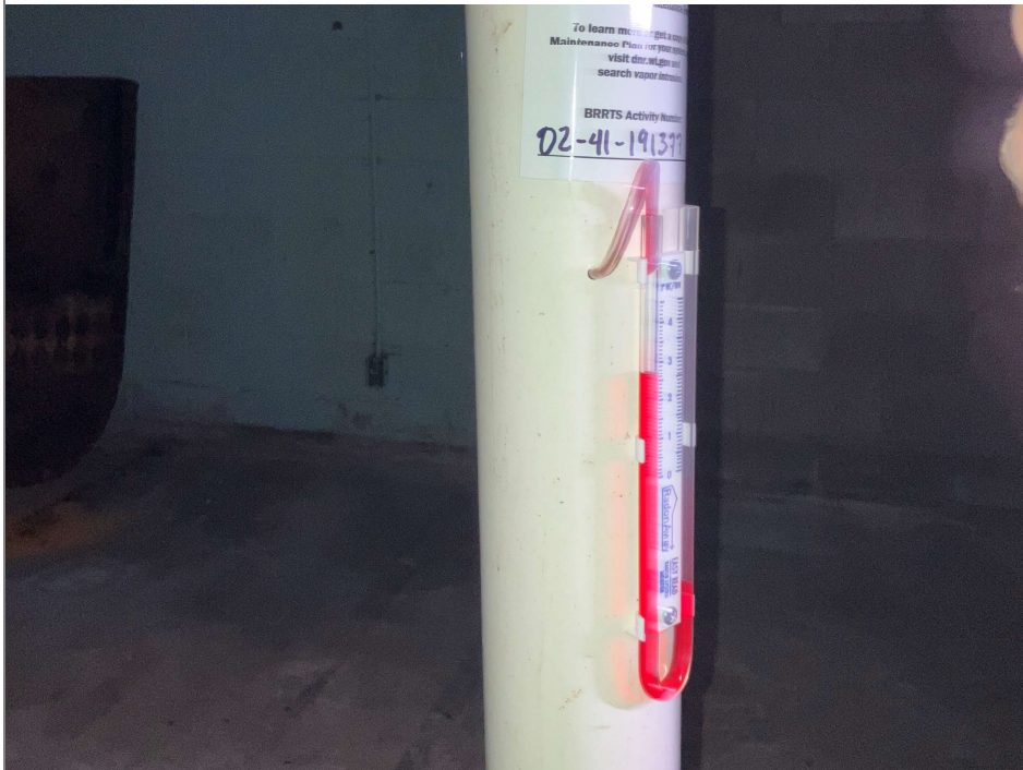
Title: VMS manometer operating properly.
