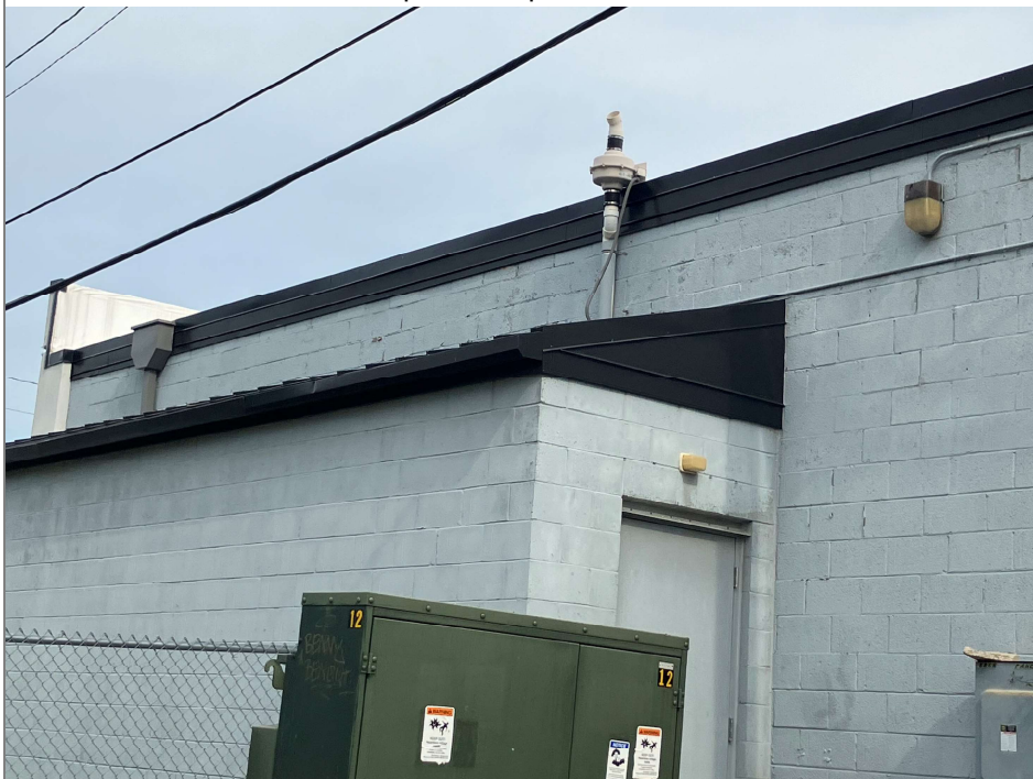
Title: Exterior fan for VMS operating.
