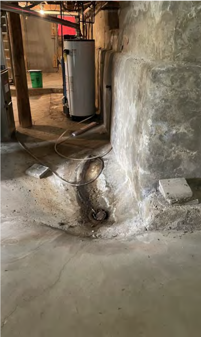
Photo 1: One floor drain located within the west side of the basement. Photograph taken on May 19, 2023.
