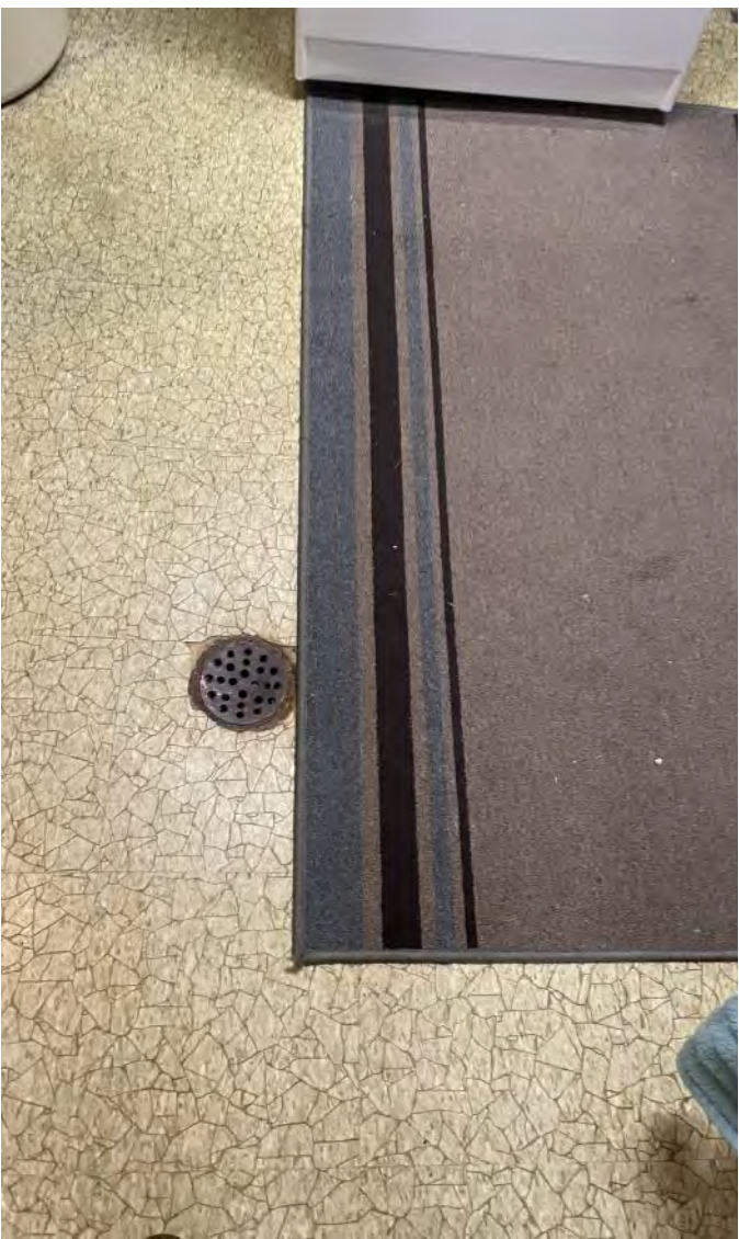
Photo 2: Floor drain within east portion of the basement. Photograph taken on May 19, 2023.
