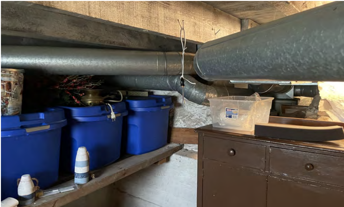
Photo 1: Indoor air sample located on the south side of the basement. Photograph taken on June 12, 2023.
