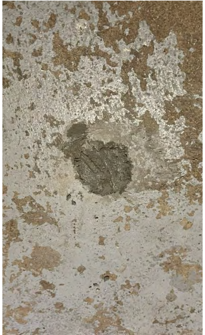
Photo 8: Abandonment of sample point near the floor crack. Photograph taken on February 16, 2024.
