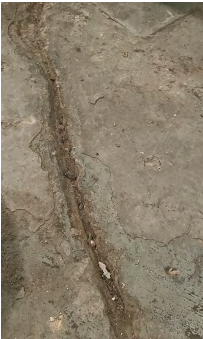
Photo 3: Crack in the floor within the basement. Photograph taken on May 19, 2023.
