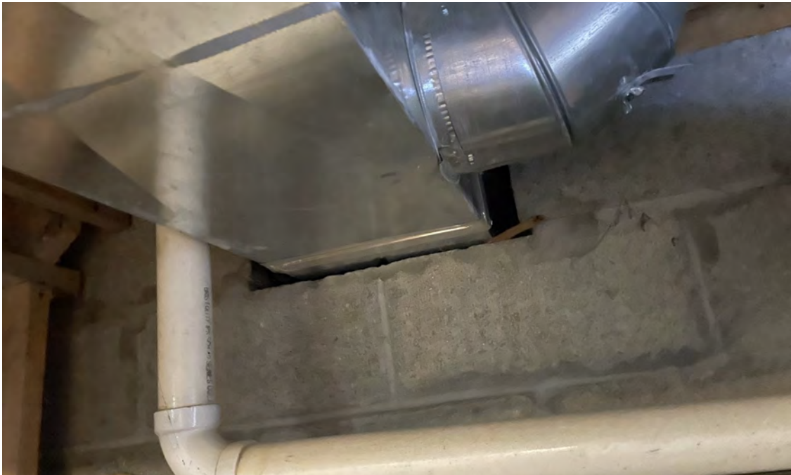
Photo 3: HVAC supply duct entering the crawlspace. Photograph taken on May 22, 2023.
