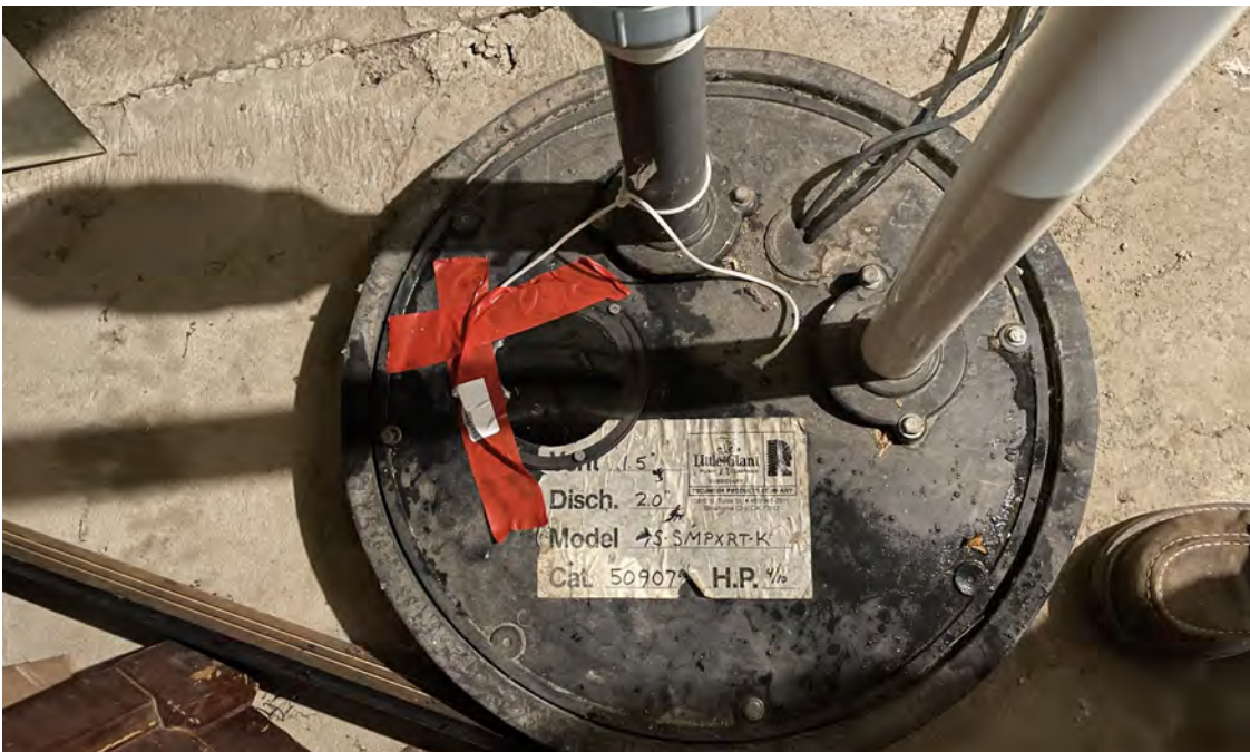
Photo 4: Sump headspace sample collected from within the sump located in the basement. Photograph taken on June 12, 2023.
