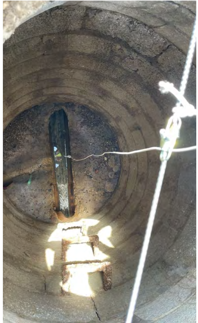
Photo 4: Sanitary sewer manhole sampler placement within the middle manhole (104). Photograph taken on June 9, 2023.
