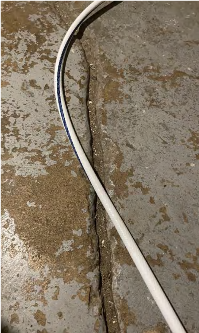
Photo 1: Crack within the basement floor located to the north of the staircase. Photograph taken on May 19, 2023.
