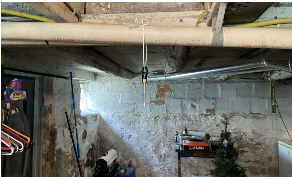
Photo 1: Indoor air sampler located on the south side of the basement. Photograph taken on June 9, 2023.
