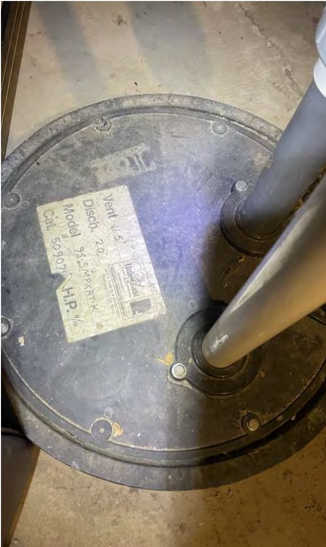
Photo 1: Basement sump with sealed cover located within the east side of the basement. Photograph taken on May 22,
