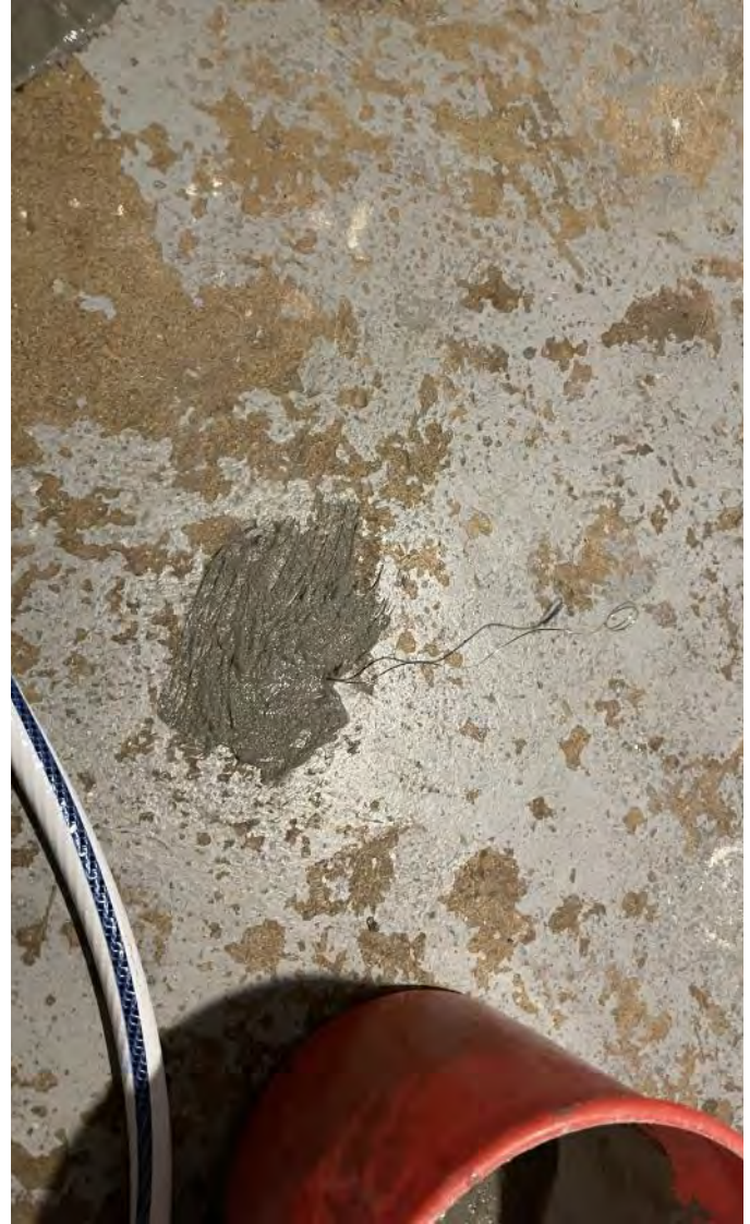
Photo 4: Temporary cement seal installed over the sample point located near the floor crack. Photograph taken on June 12, 2023.
