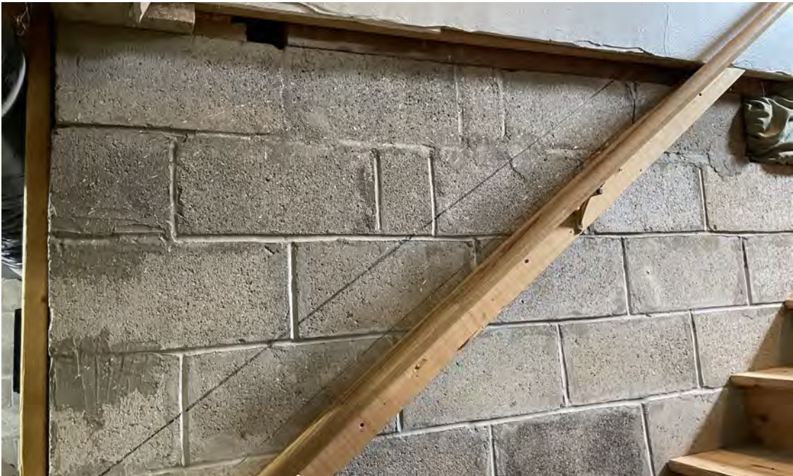
Photo 4: Block wall within the basement with the crawlspace on the other side. Holes were observed within the block wall. Photograph taken on May 22, 2023.
