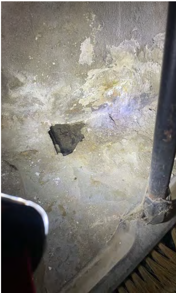
Photo 1: Hole in floor within the basement. Photograph taken on May 19, 2023.
