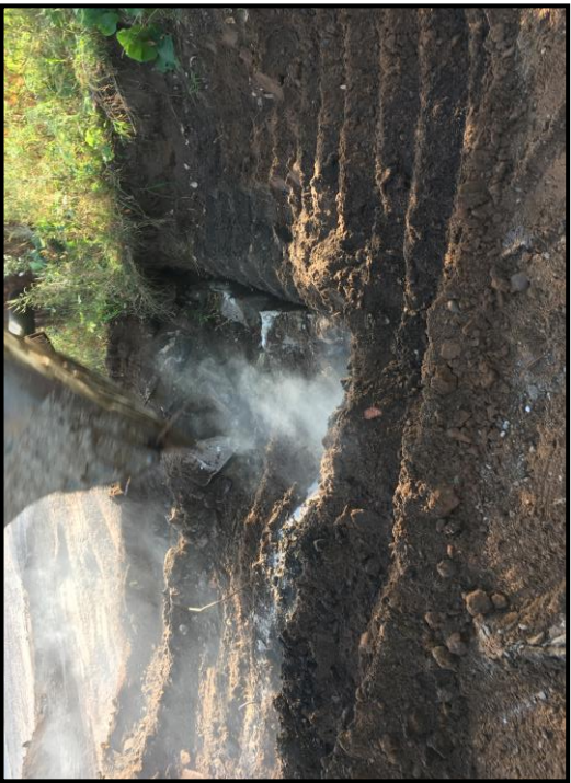
Concrete discovered during excavation
