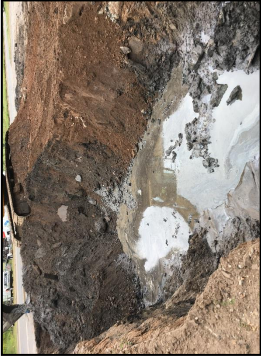
Water in excavation, west side
