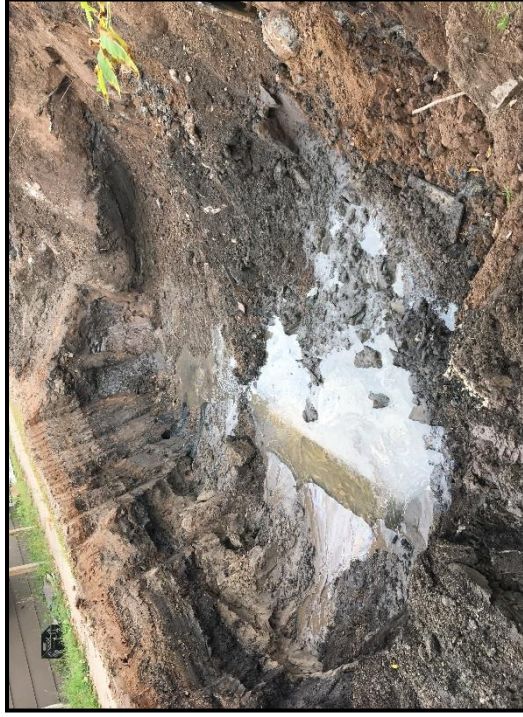
Water infiltrating from western sidewall
