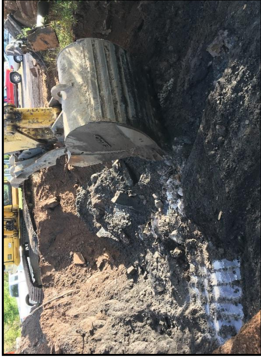
Some groundwater infiltrating excavation, additional concrete rubble
