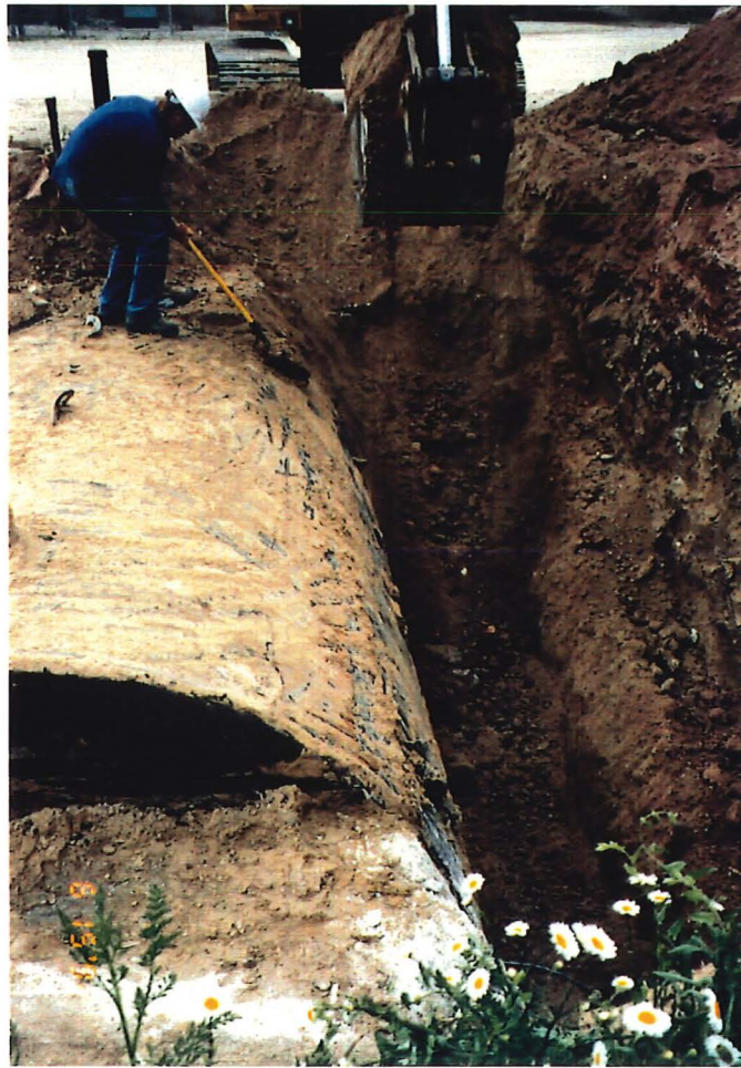
Description 11K tank Date 06/15/92 Customer Tecumseh Products Photo # 6-7 Camera Setting auto Project # 15292 Project Manager William Fisher
