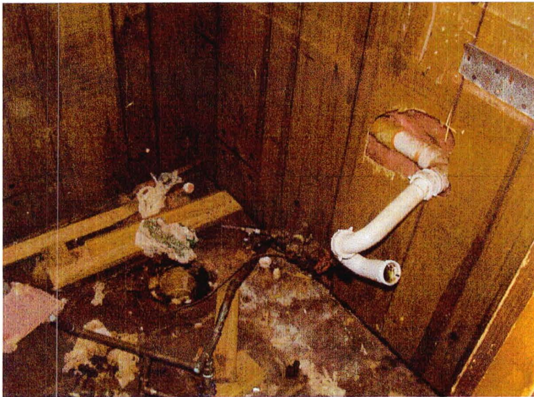
Disconnected bathroom plumbing
