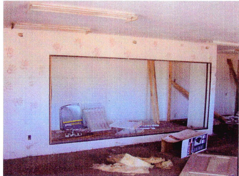
View of cooler area
