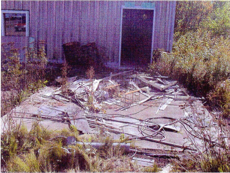
Debris on concrete pad, outside southwest building entrance
