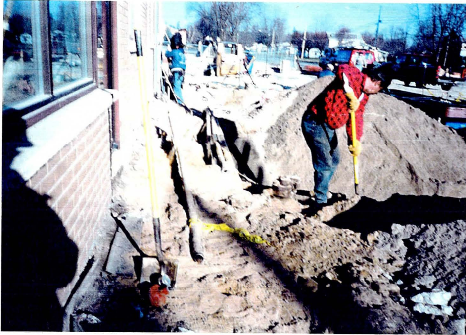
PHOTO 1 View of the product and vent piping along the east side of the building.
