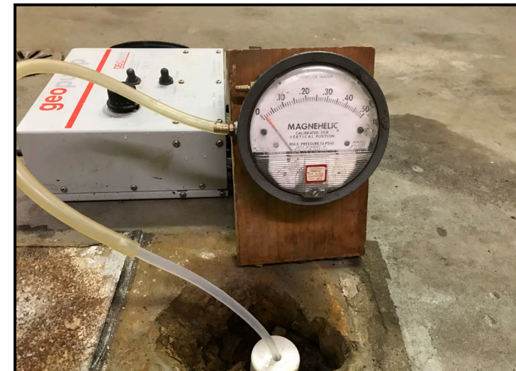
No measureable vacuum at TW1400
