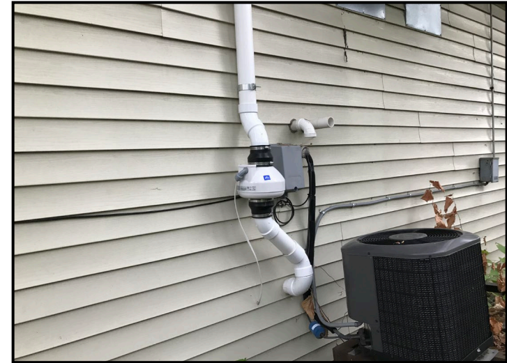
Vapor mitigation system - exterior
