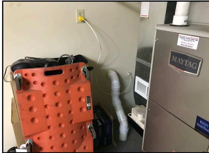
Vapor mitigation system in western storage area
