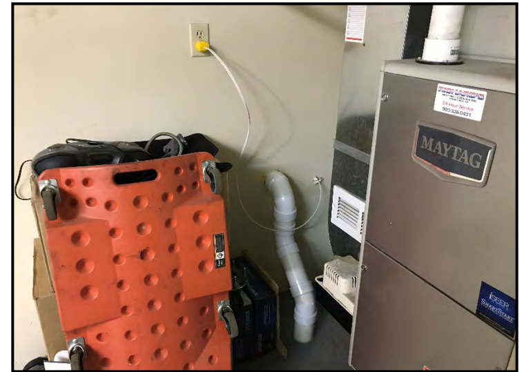
Vacuum point and power source
