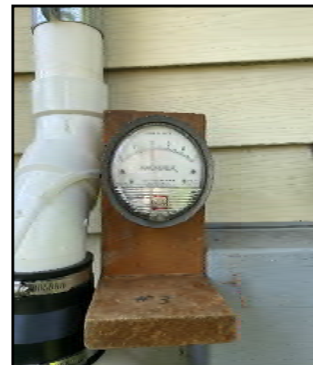
2" of water column
