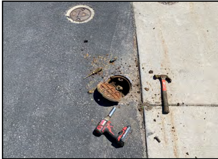
SVE-2, MW800 in background
