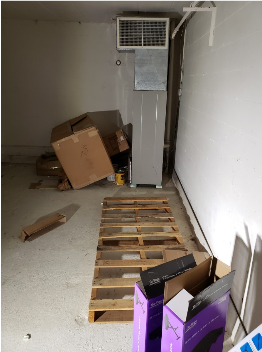
Photo 21: Heating unit in Jim's Annex basement (4/2/20; 13:57).
