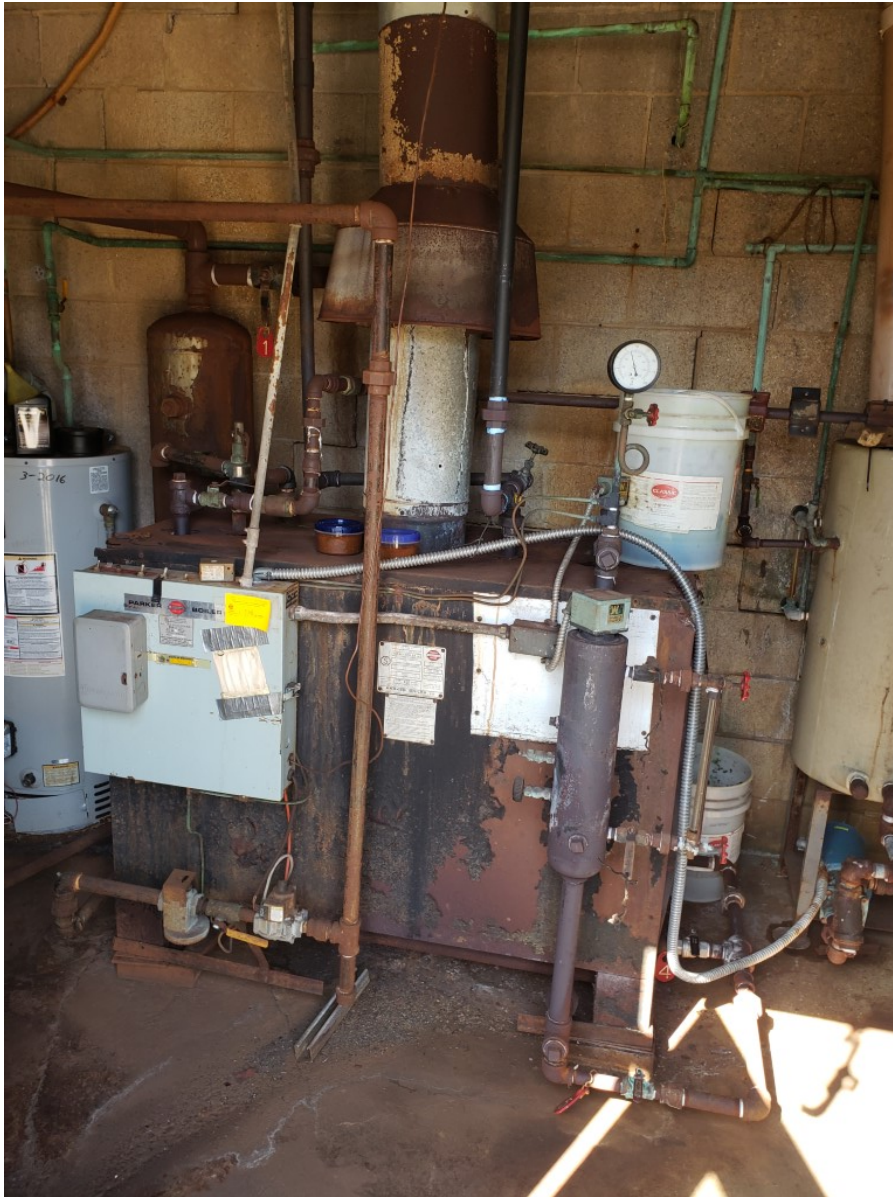
Photo 8: Boiler at back of dry cleaner (unit 1233), (4/2/20; 11:13).
