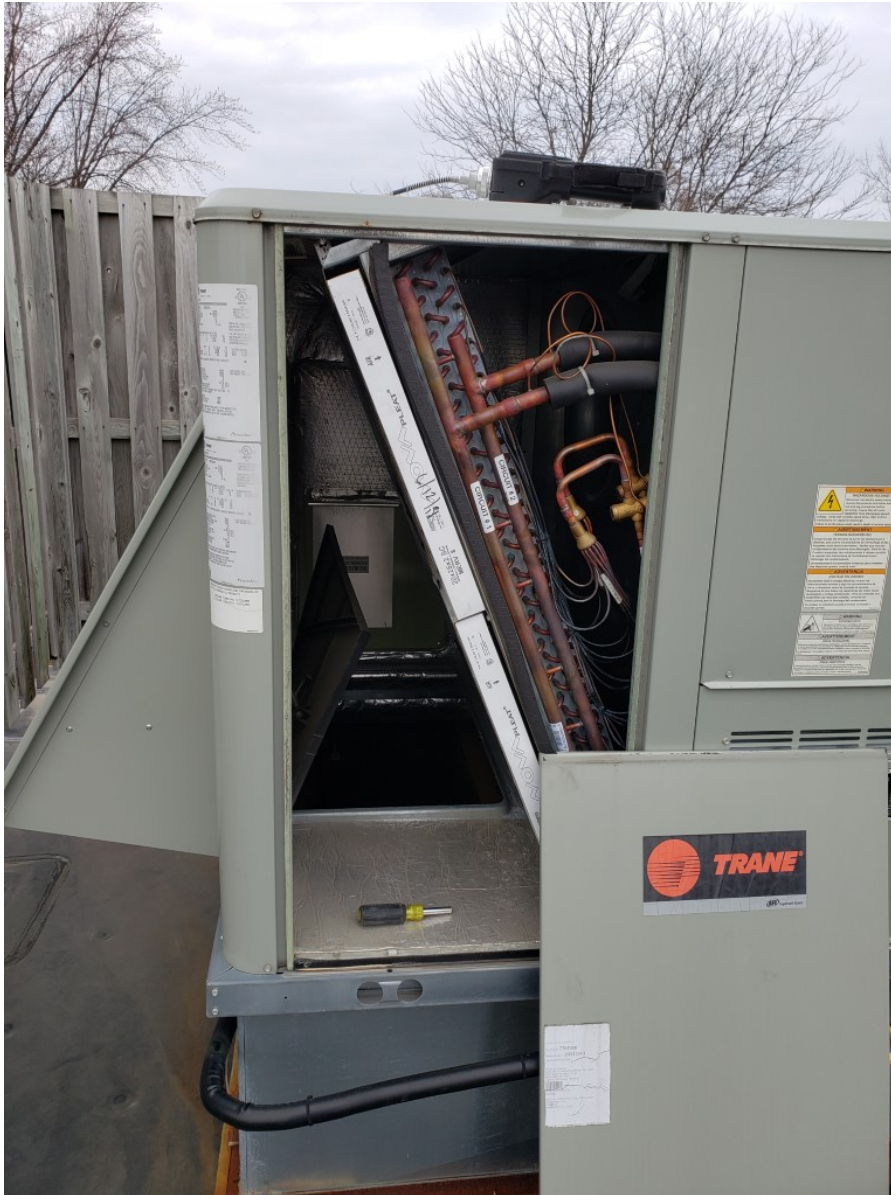
Photo 32: Roof-top HVAC unit at Jim's (unit 1219) showing damper for indoor return air (4/3/20; 14:45).
