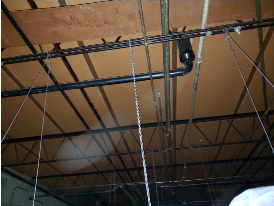
Photo 11: Interior view of plumbing vent with high PID result, Jim's Music (4/2/20; 12:30).
