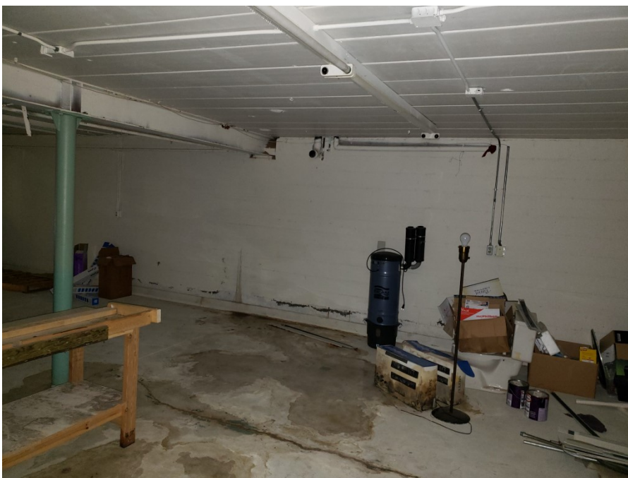
Photo 19: Water on floor in basement of Jim's annex (4/2/20; 13:52).
