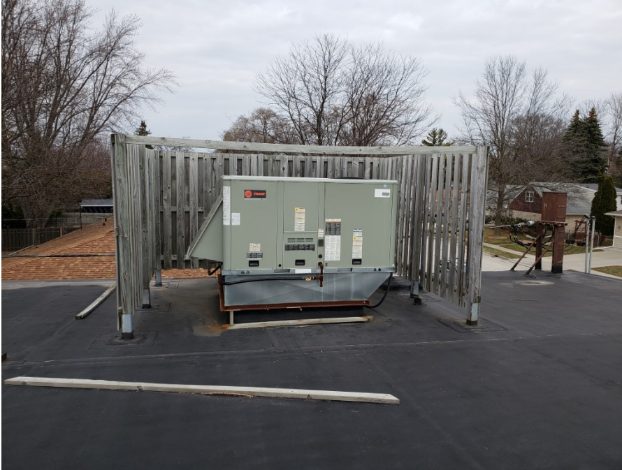
Photo 33: Roof top HVAC unit on Jim's Music (4/3/20; 14:55).
