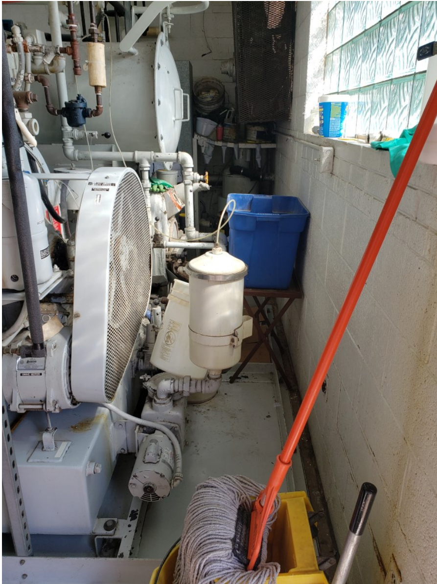
Photo 7: Back of dry cleaning machine in unit 1233 (4/2/20; 11:13).
