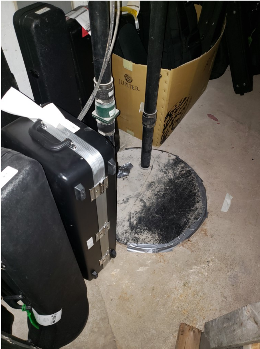
Photo 13: Sump at back wall of Jim's basement adjacent to water and sewer connections to street (4/2/20; 12:34).
