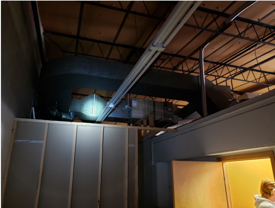
Photo 16: HVAC unit in ceiling of Jim's annex (4/2/20; 13:34).
