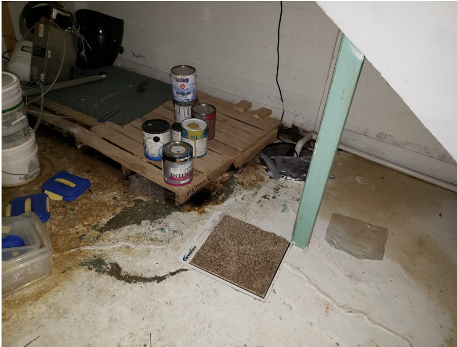
Photo 18: Sump near NE corner of Jim's annex basement (4/2/20; 13:53).
