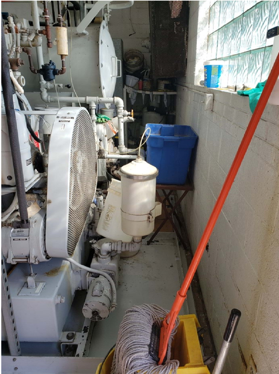
Photo 7: Back of dry cleaning machine in unit 1233 (4/2/20; 11:13).
