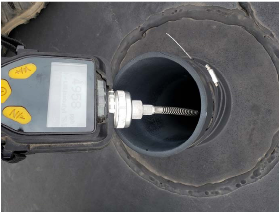
Photo 31: Plumbing vent in roof of 1219 unit with elevated PID reading (4/3/20; 14:36).
