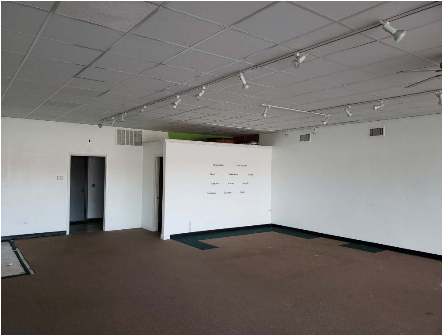
Photo 5: Former Williams Tae Kwon Do (unit 1235) back and south walls with HVAC vents near ceiling (4/2/20; 10:50).
