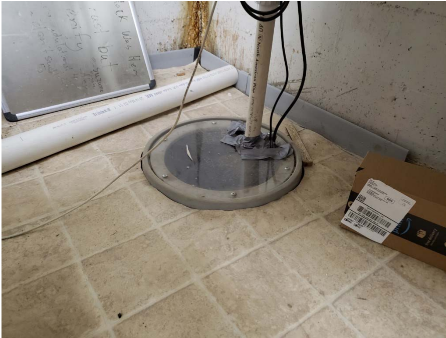
Photo 14: Sump at NW corner of Jim's basement in office area (4/2/20; 12:51).
