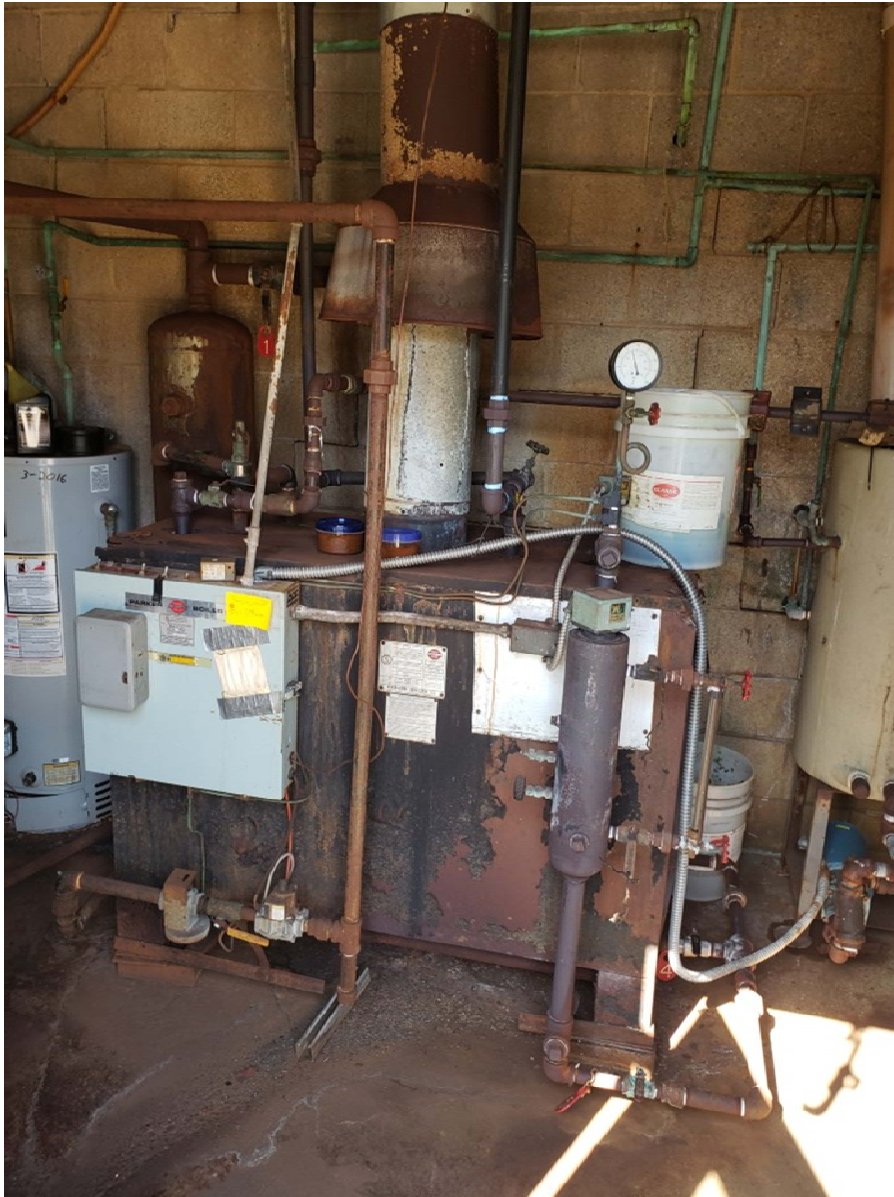
Photo 8: Boiler at back of dry cleaner (unit 1233), 4/2/20; 11:13.
