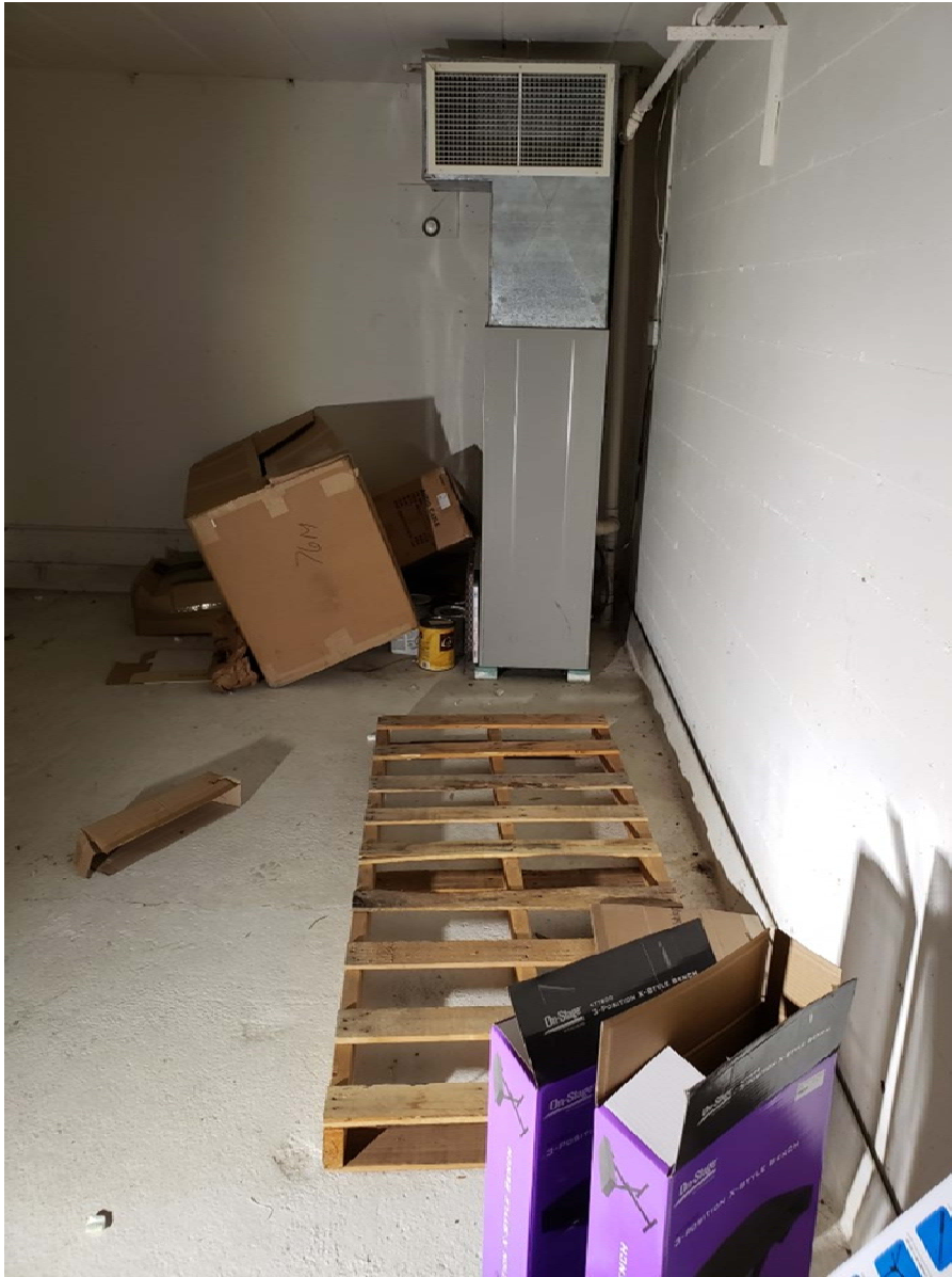
Photo 21: Heating unit in Jim's Annex basement (4/2/20; 13:57).
