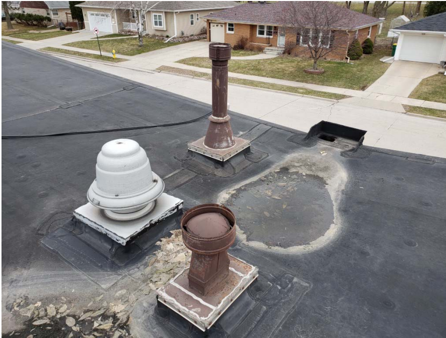
Photo 30: Bathroom fan vents (rusty) and basement exhaust fan (gray) at common wall between 1231 and 1219 units (4/3/20; 14:32).
