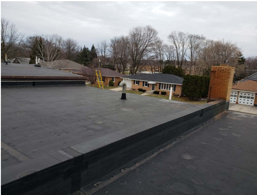
Photo 27: Roof of dry cleaner showing boiler room chimney and cleaning machine vent (galvanized pipe), (4/3/20; 14:30).
