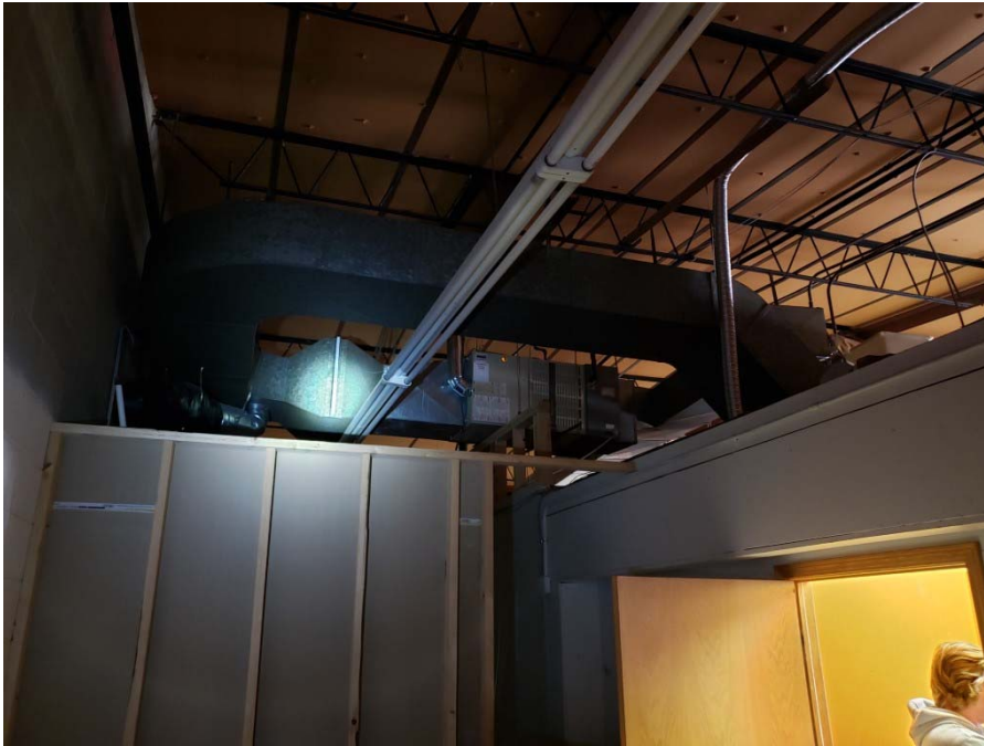
Photo 16: HVAC unit in ceiling of Jim's annex (4/2/20; 13:34).
