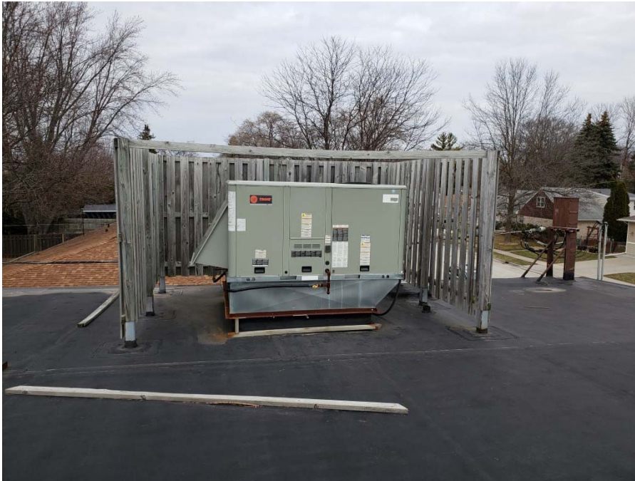
Photo 33: Roof top HVAC unit on Jim's Music (4/3/20: 14:55).
