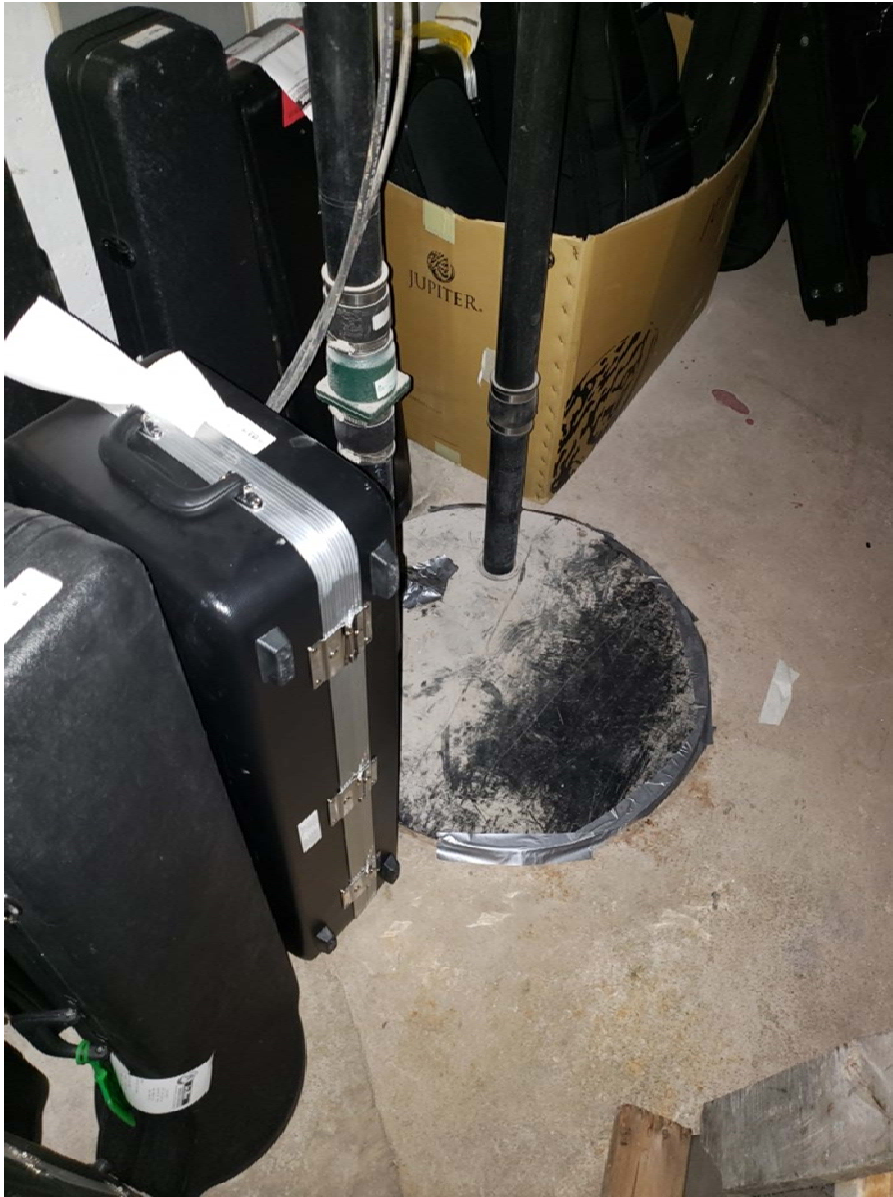
Photo 13: Sump at back wall of Jim's basement adjacent to water and sewer connections to street (4/2/20; 12:34).
