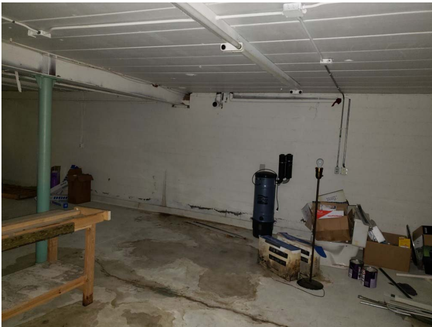
Photo 19: Water on floor in basement of Jim's annex (4/2/20; 13:52)
