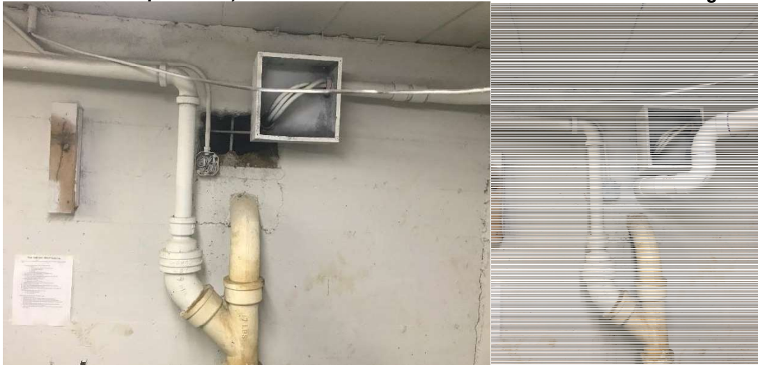
Photo 10. Vacuum extraction points P7, west wall of north basement. Before and after sealing.
