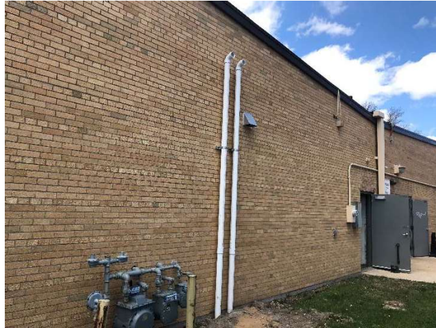
Photo 17. Discharge vents from north basement.
