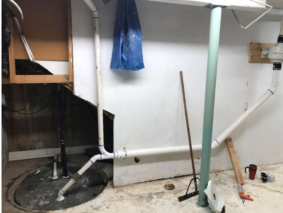
Photo 9. Vacuum blower B3, south basement sumps.
