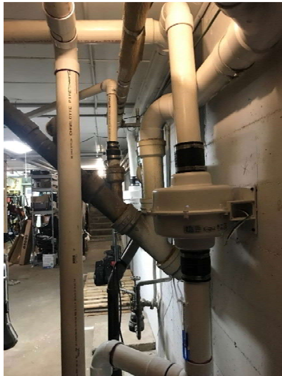
Photo 12. Vacuum extraction blower B2, north basement.
