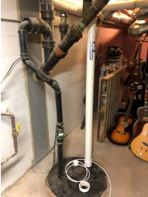
Photo #7 View of Sump 2 and differential pressure gauge facing southwest.
