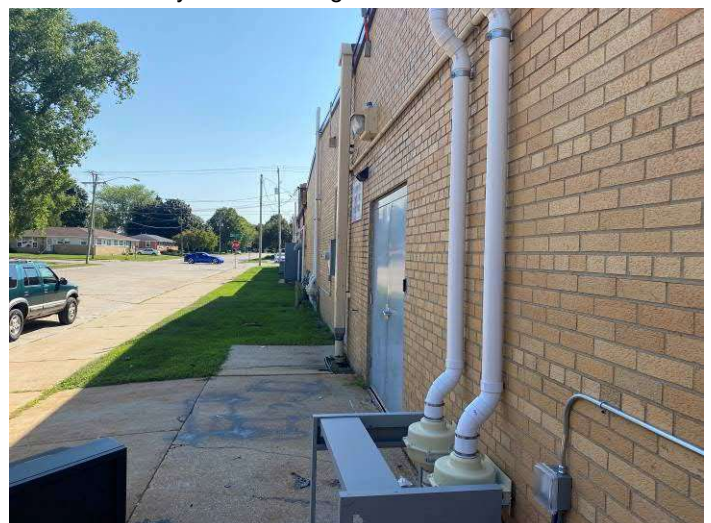
Photo #6 General view of exterior systems at B1 and B2 facing southwest.
