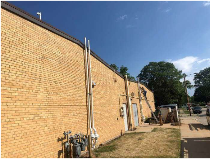
Photo #1 View of outdoor vent piping and fans located at back of building facing northwest.
