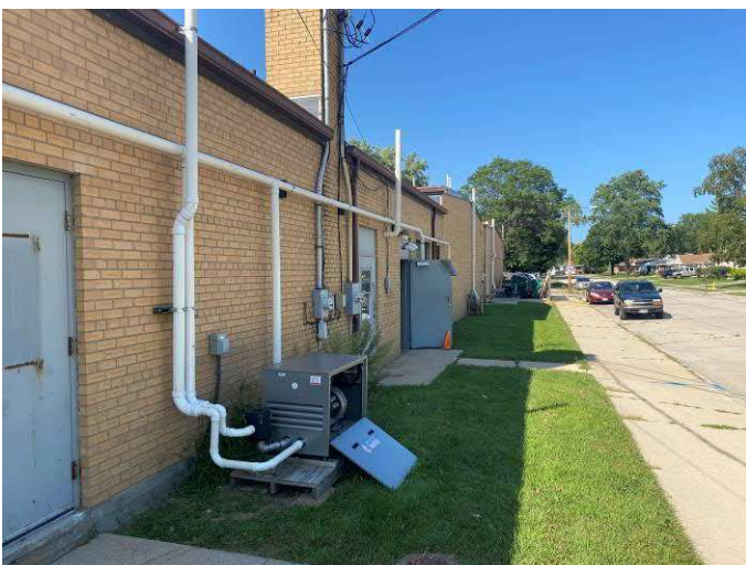
Photo #5 View of blower and outdoor vent piping facing northwest.
