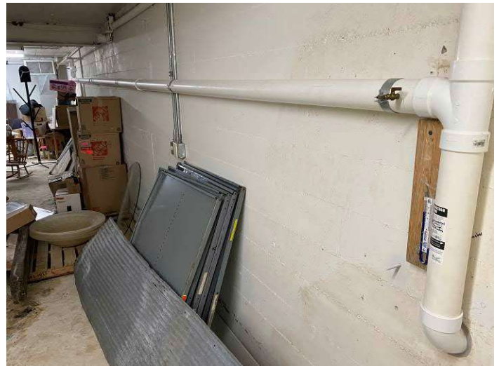
Photo #4 View of differential pressure gauge and collection piping at System B4 facing south.
