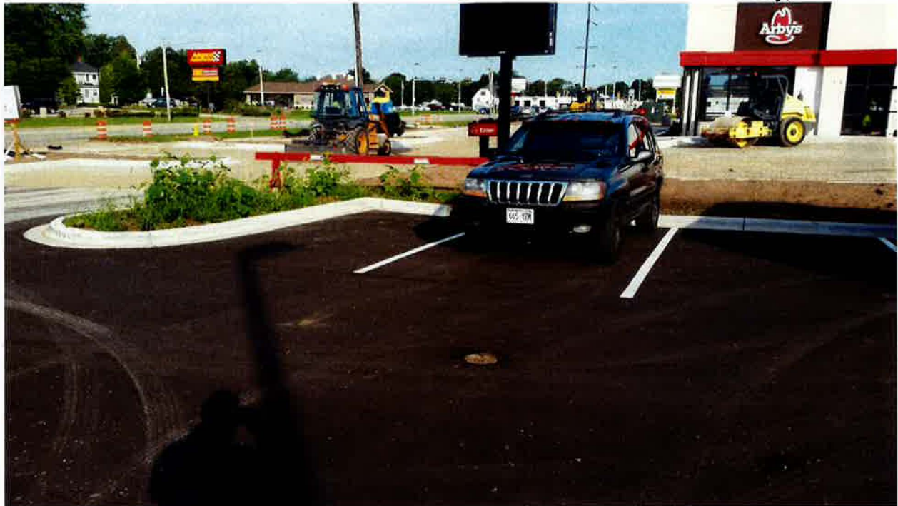
PHOTOGRAPH OF PAVED AREA AROUND MW-3 VIEWING TOWARD THE WEST AND THE ADJOINING ARBY'S CONSTRUCTION
