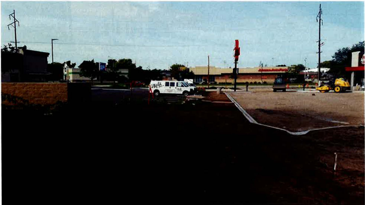
PHOTOGRAPH OF THE BERM AREA VIEWING FROM THE NORTHWESTERN PORTION OF THE PROEPRTY TOWARD THE SOUTHWEST
