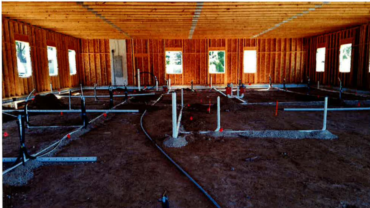
PHOTOGRAPH OF VAPOR MITIGATION SYSTEM PIPING AND OTHER BUILDING PLUMBING VIEWING FROM THE NORTHWEST TOWARD THE SOUTHEAST
