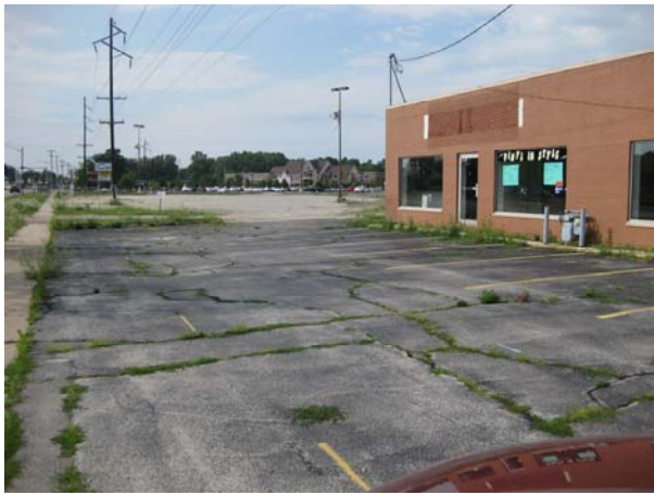
Photo 1: Pre building demo front side of building, face North from near MW-8 (July 2012)
