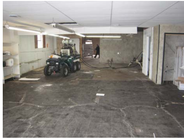
Photo 4: Pre building demo inside drilling, face Northeast from near west building corner (December 2012)
