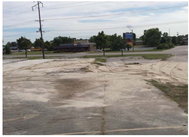
Photo 8: Remedial Excavation, final dig limits and backfilled, face Southwest from near MW-4 (August 2015)
