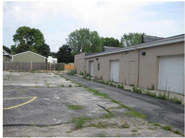
Photo 2: Pre building demo loading docks back side of building, face Southeast from near MW-4 (July 2012)
