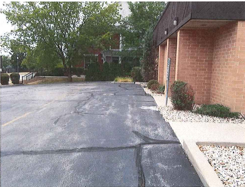
Looking south at the asphalt cap east of the dry clean facility
