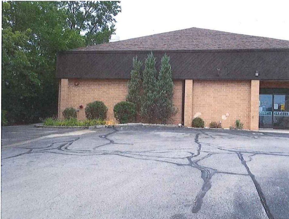
Looking west at the asphalt cap (MW-5 is located in the center right of the photo)
