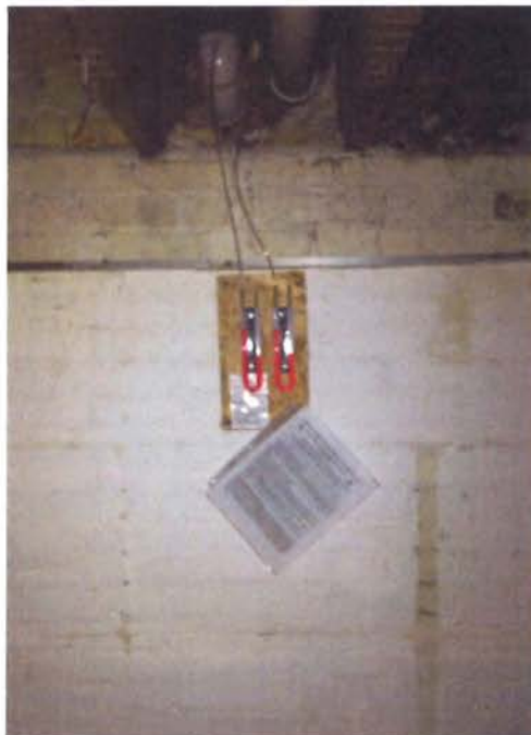
Photo 14: Manometers, label, operation & maintenance information, and warranty information
