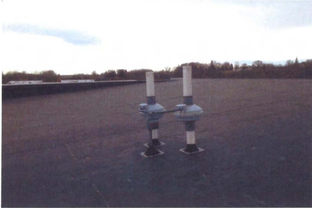
Photo 15: Fans above roof
