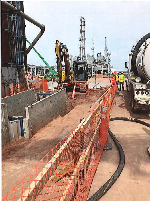
Title: Looking north at capped area. Cap begins on at the edge of concrete on the east side of trench box. SRC is sampling soil being excavated for the utility trench.
