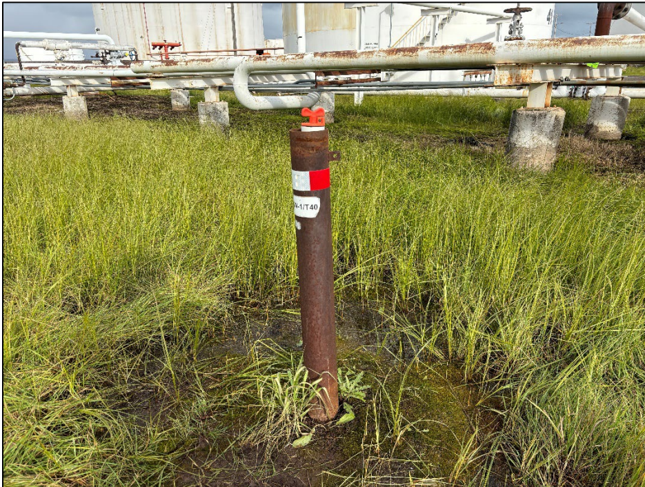
Photo 2: MW-1/T40 after riser and was replaced. Photo taken November 7, 2023.
