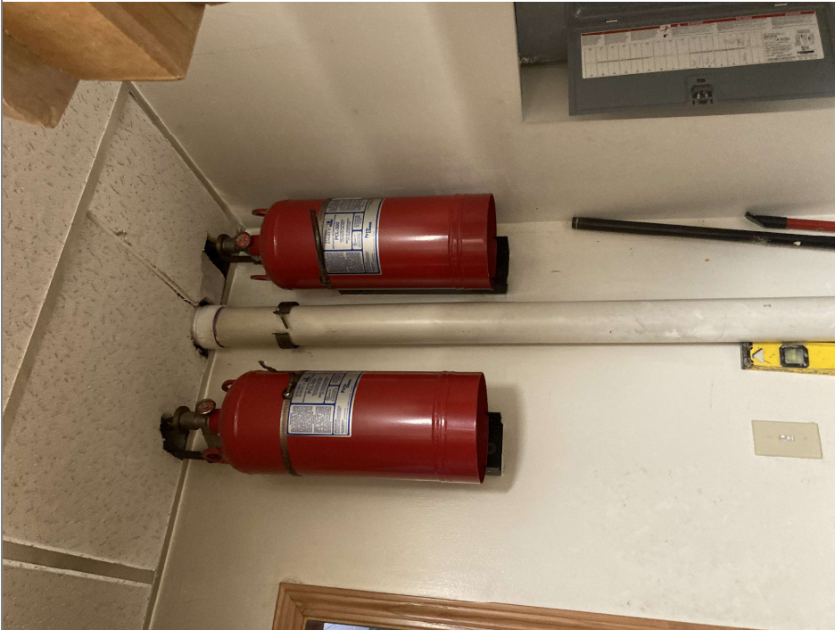
Title: Paul's Classic Cleaners, 02-13-227101: Riser pipe & location of former manometer 09/13/2023
