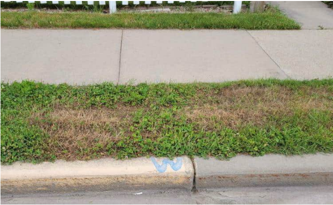
Location of boring B-7 in the terrace to the left of the water lateral.
