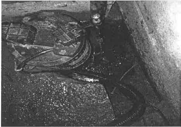
Sump pump/sump pit
