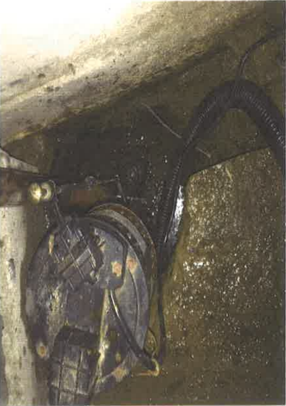
Sump pump/sump pit
