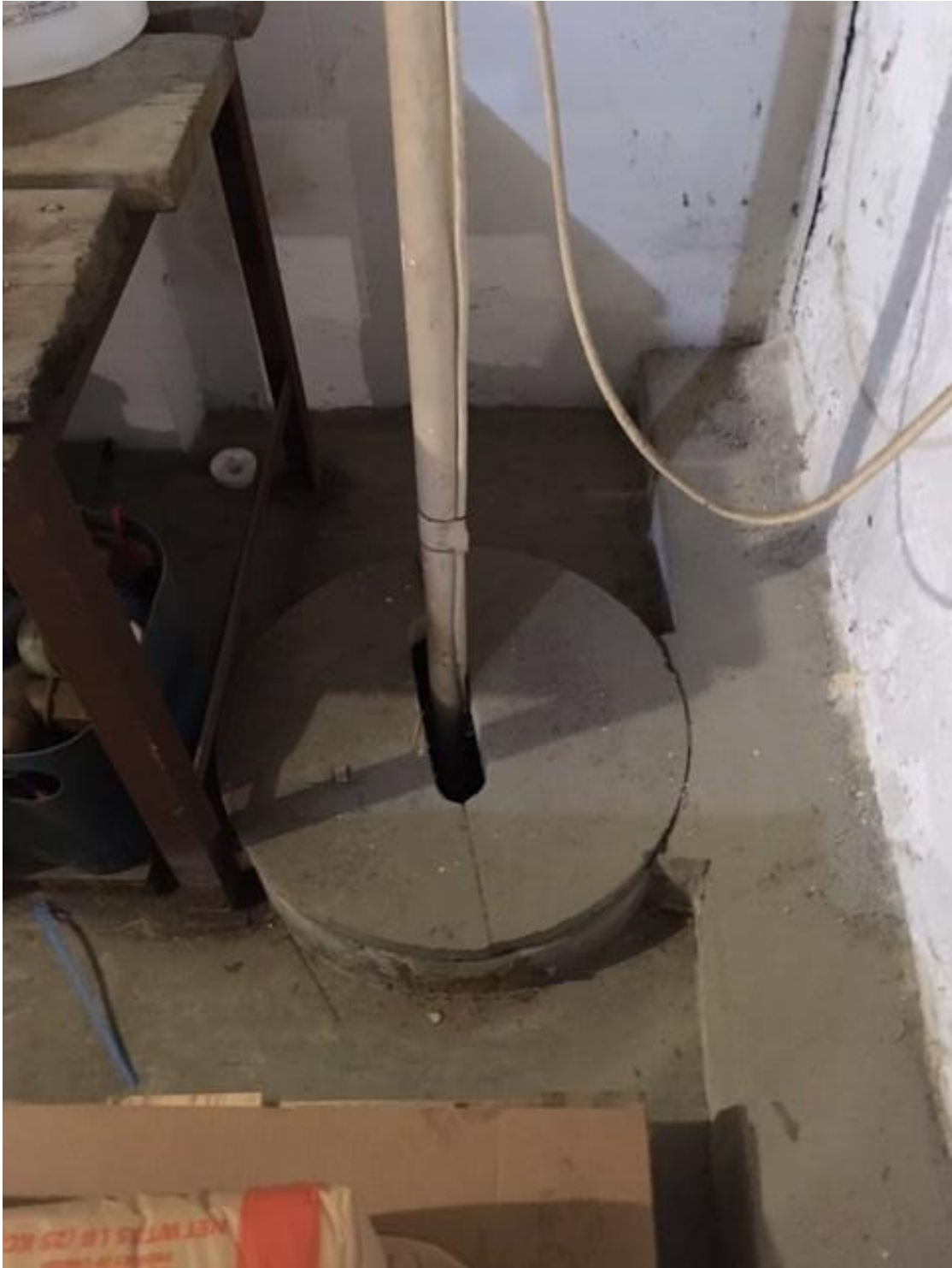
Photo 1: Sump Pump – Milwaukee Plating
