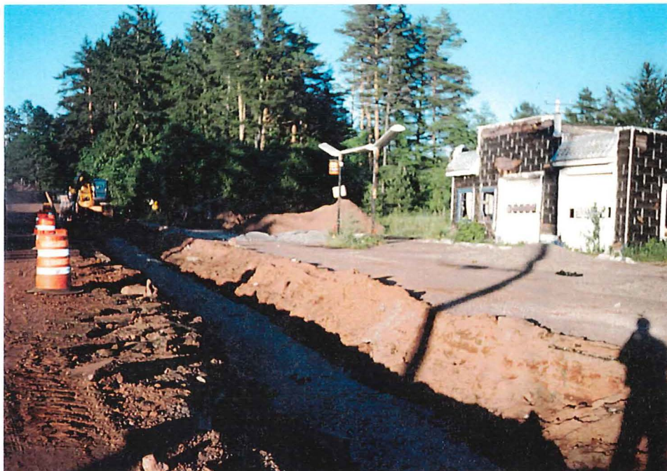
Photograph #2: View of the former Thomas service station with the installed storm sewer (facing southeast).
