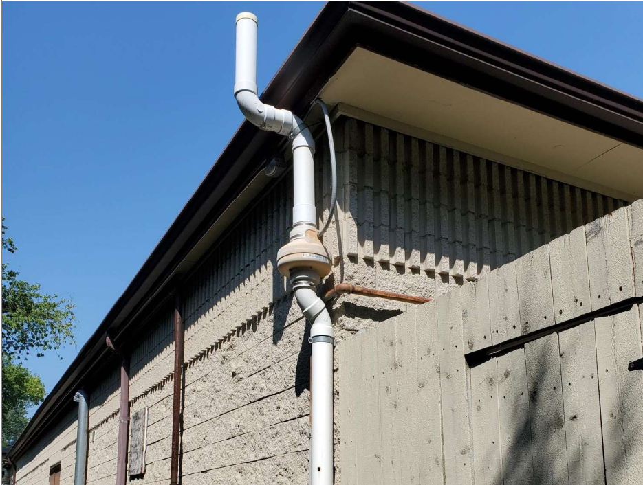
Title: Mitigation fan - southeast corner of building
