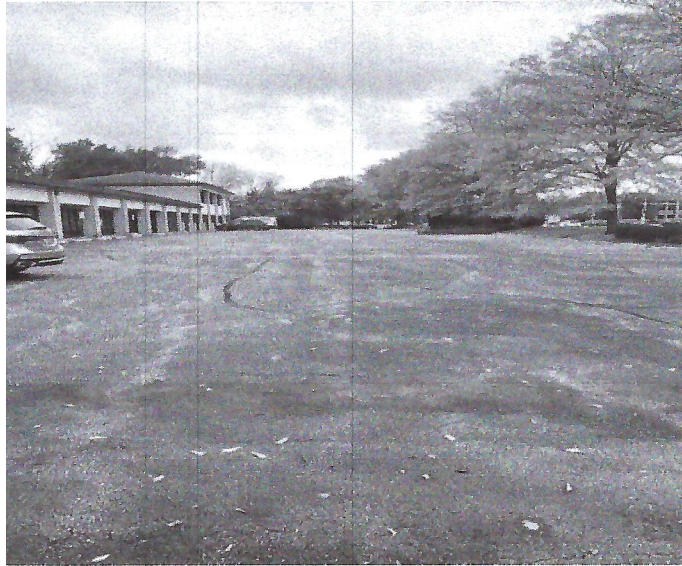
Photo 1 Looking west at existing asphalt cover between the existing building and W. North Ave. Pavement appears to be in good condition with no signs of deterioration or exposed soil.
