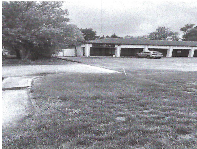
Photo 3. Looking south at existing asphalt pavement. Pavement appears to be in good condition with sign of deterioration or exposed soil.
