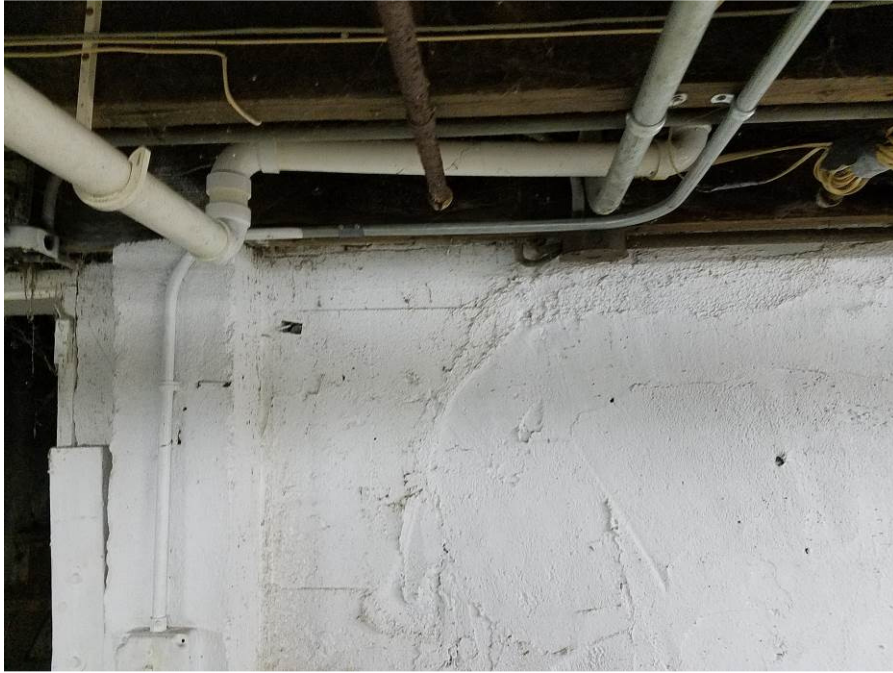
Photo 5: Sump pump piping at east end of building
