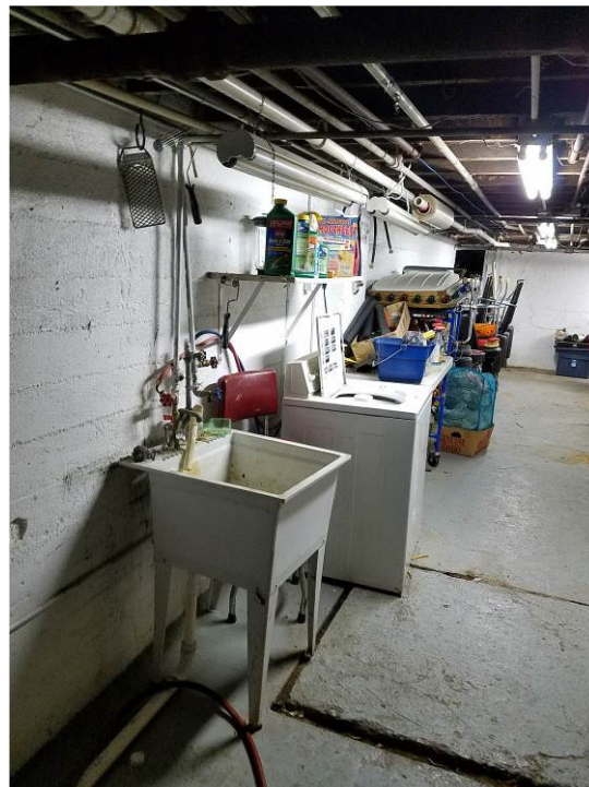
Photo 2: Looking east at sump pump piping in rafters
